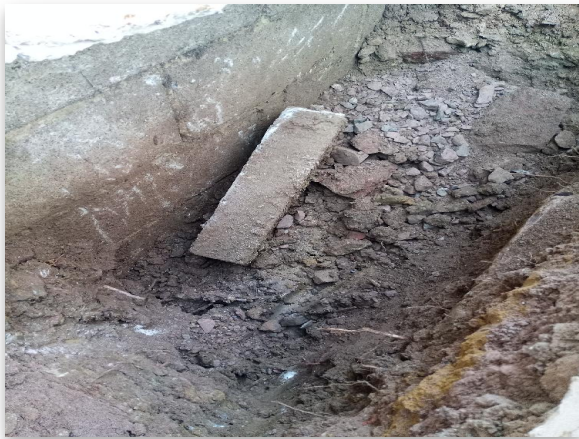
Fig 2.3: Rubble within Hole
