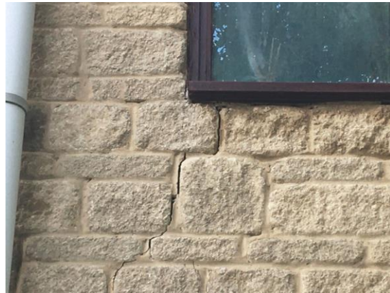
Cracking below bathroom window.
