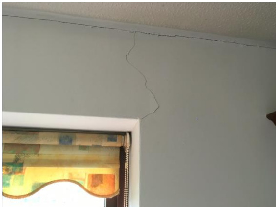
Cracking above kitchen window.
