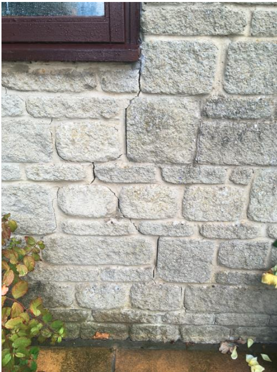
Cracking below kitchen window.
