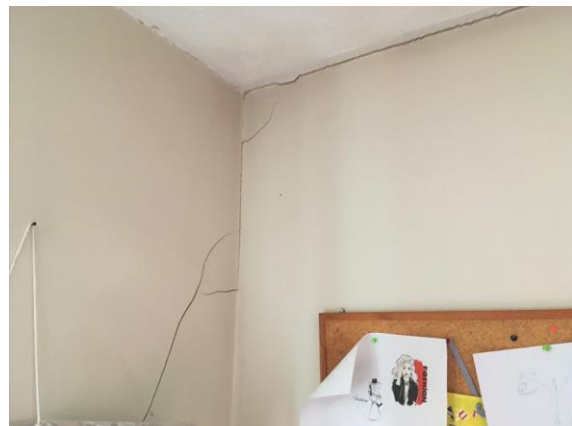
Cracking to bedroom
