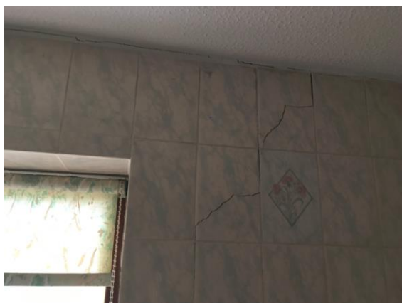
Cracking to bathroom
