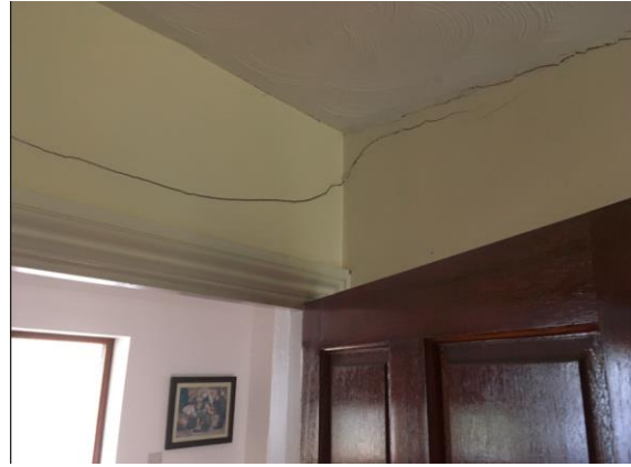
Cracking above office door head..
