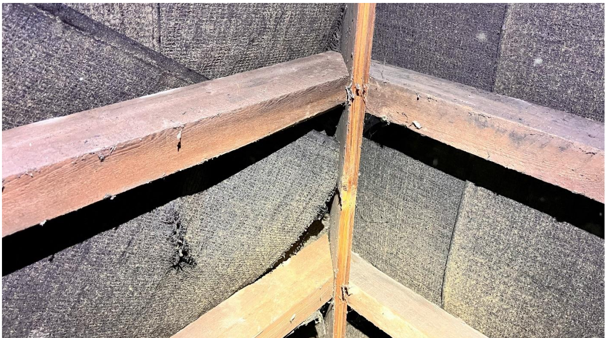
Photograph 4: The section of bitumen felt adjacent to the ridge board which has sagged, beneath which the aggregation of droppings were located.
