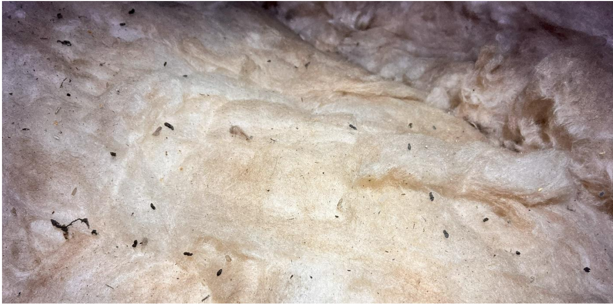
Photograph 3: Dropping evidence within the roof void.
