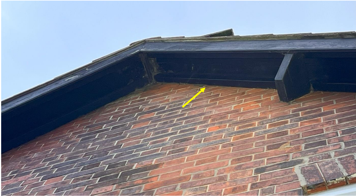
Photograph 7: Evidence of space behind exposed timber features on the gable ends and at the eaves. This image shows the western gable.
