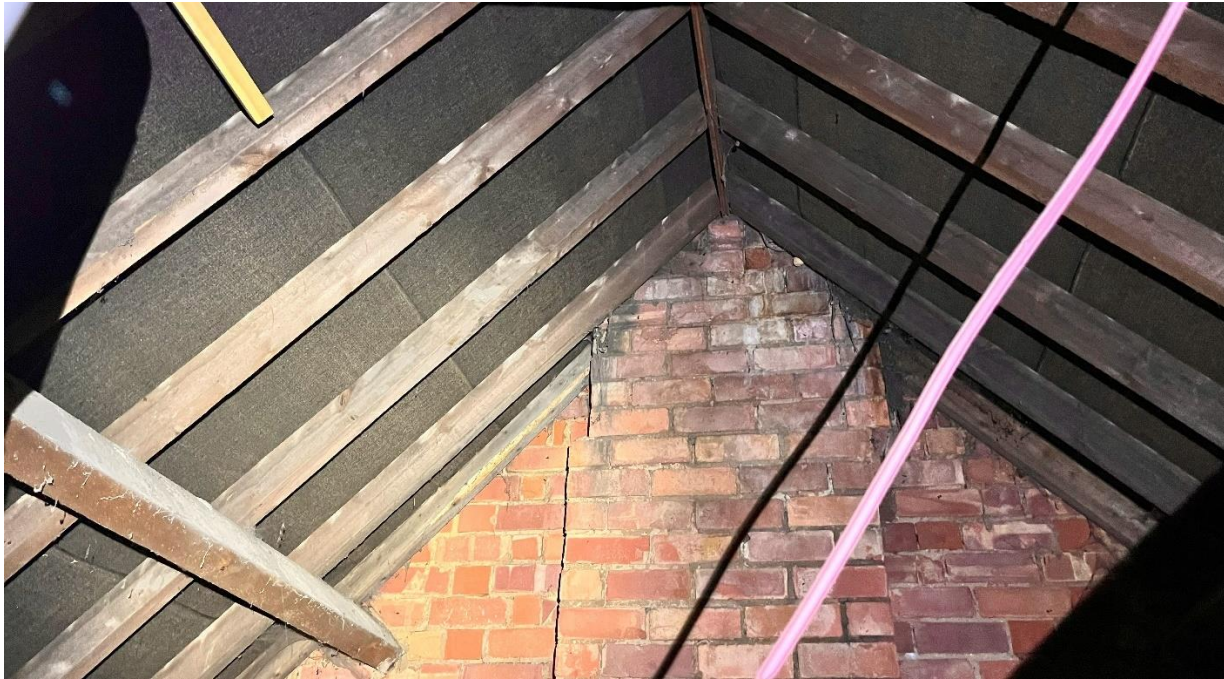
Photograph 5: The roof void of the dwelling, pointing toward the western gable of the main pitch, showing the uncluttered space, the timber frame and the bitumen felt underlining. Note the relative lack of cobwebs along the ridge.
