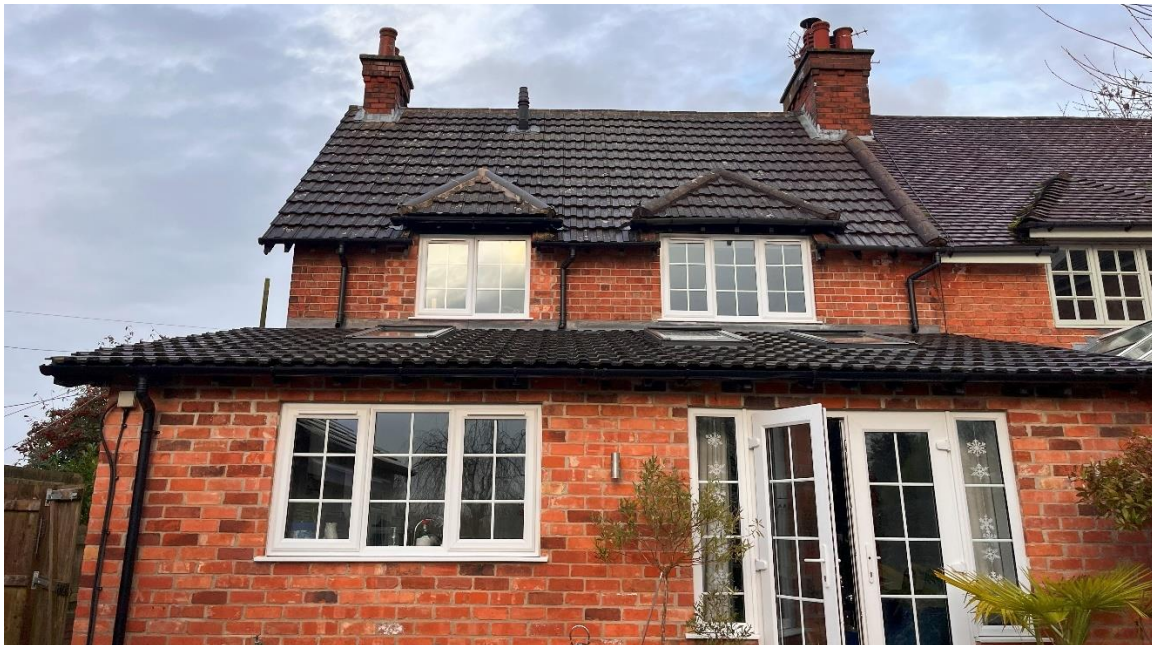
Photograph 2: 86 Caythorpe Road, taken from the south, showing the single-storey extension to the rear of the property.
