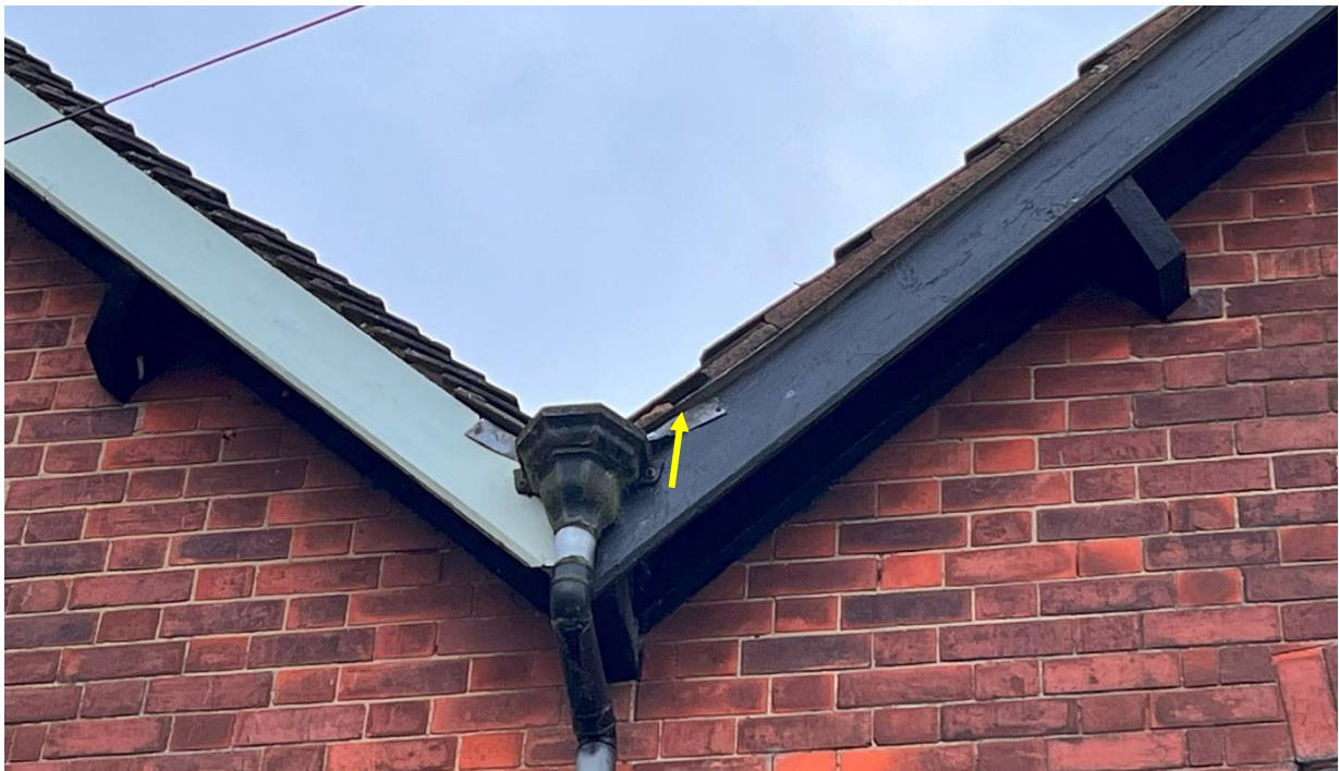
Photograph 8: Evidence of missing bedding mortar on the gable verge of the north facing extension.
