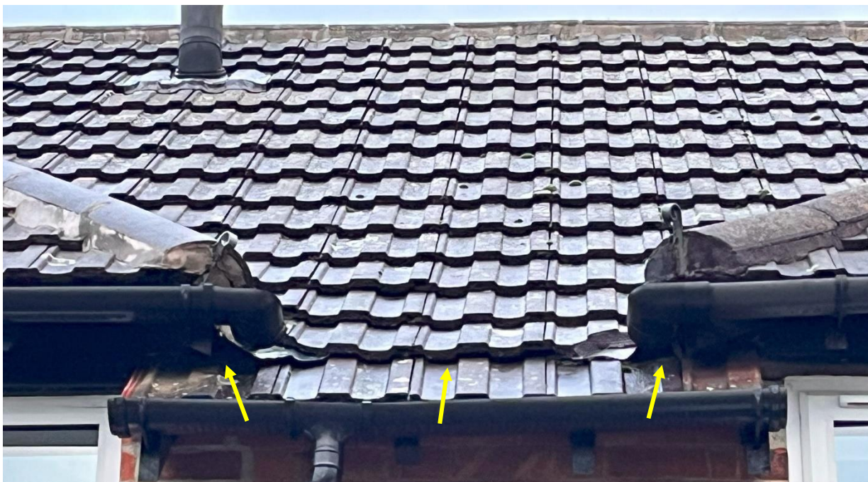
Photograph 6: Evidence of gaps beneath roof tiles and around the mini roof structures associated with the bay windows.
