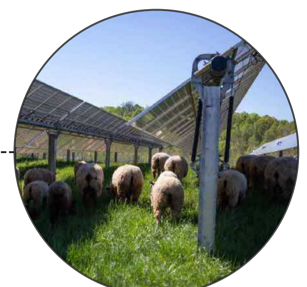
IMPROVED GRASSLAND UNDER SOLAR ARRAYS
