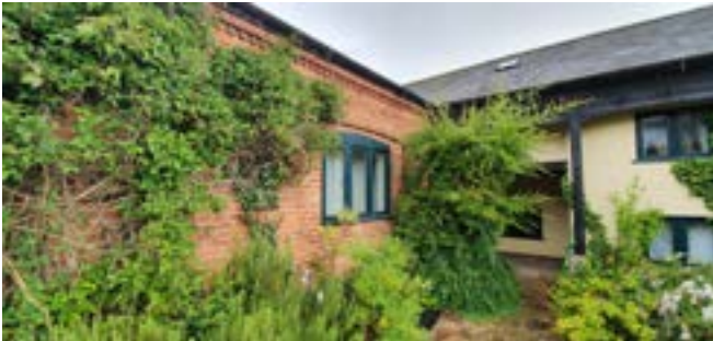
View of south facing elevation showing where original arched openings have been closed to form windows. The proposal is re-open the original arches.
