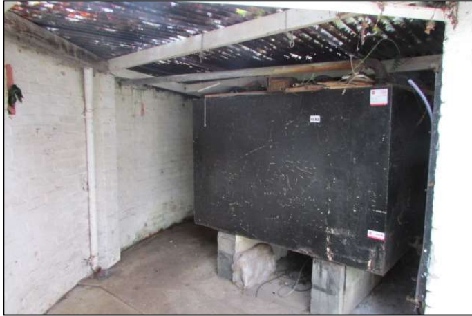
Figure 17 - Oil tank within the yard.
