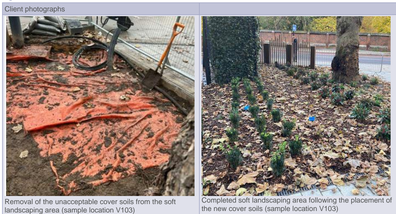
Figure 5-1 Remediation areas corrective actions
