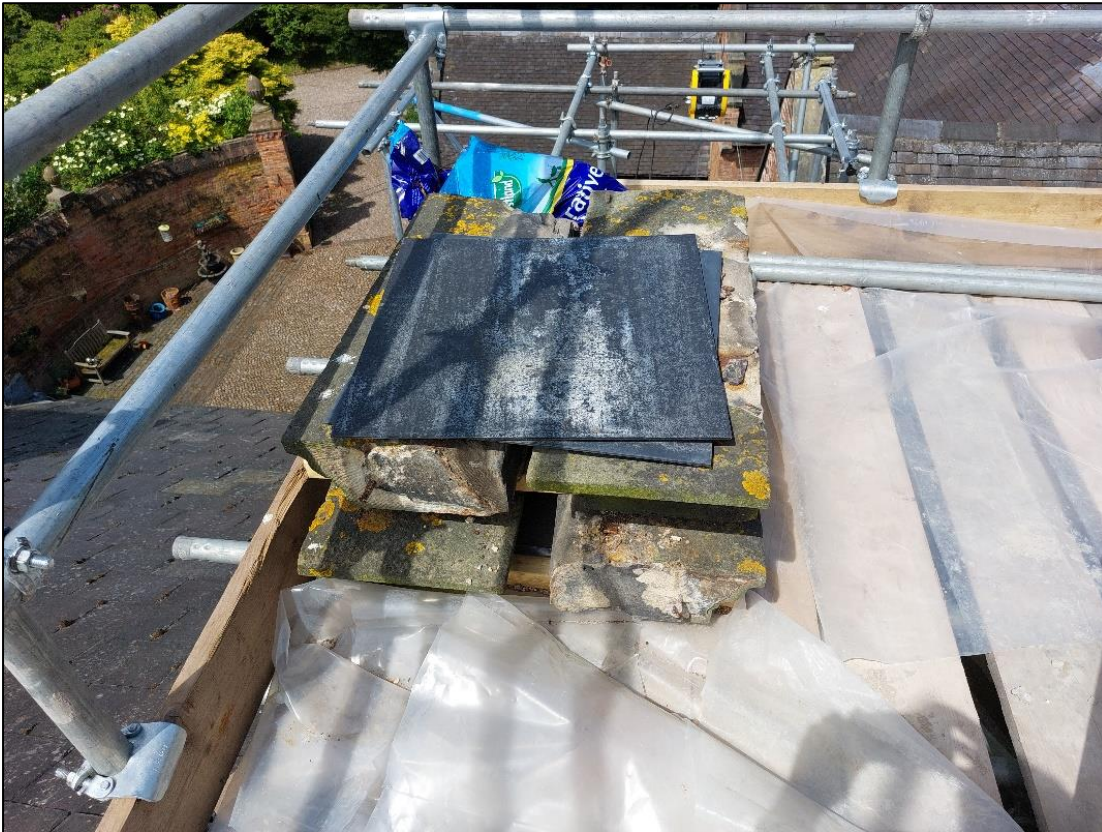
Fig.3 – Stone cornice removed to stack 1 will be reinstated. 1no. new cornice section is required.
