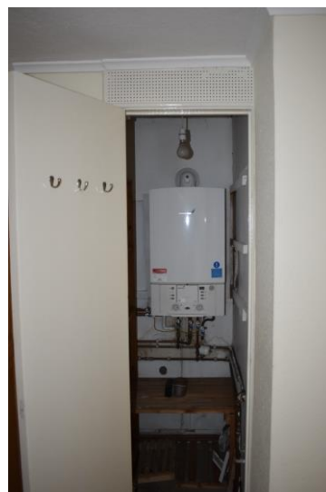
Figure 11. Boiler room on first floor
