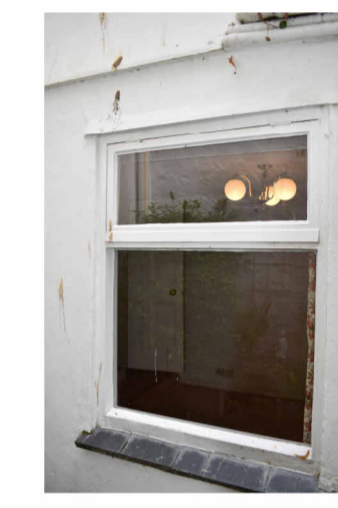
Existing Window WGF04. To be removed, no significant historic or architectural merit, frame compromised.
