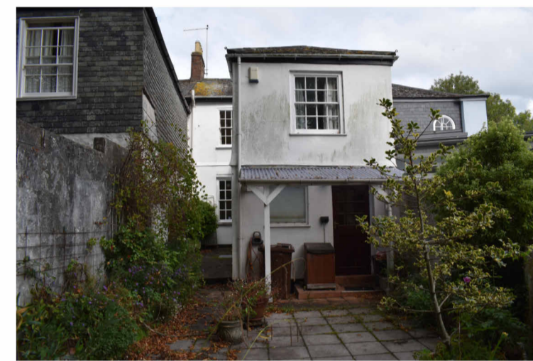
Existing Lean-to Roof (proposed to be removed) is of no historic or architectural merit.
