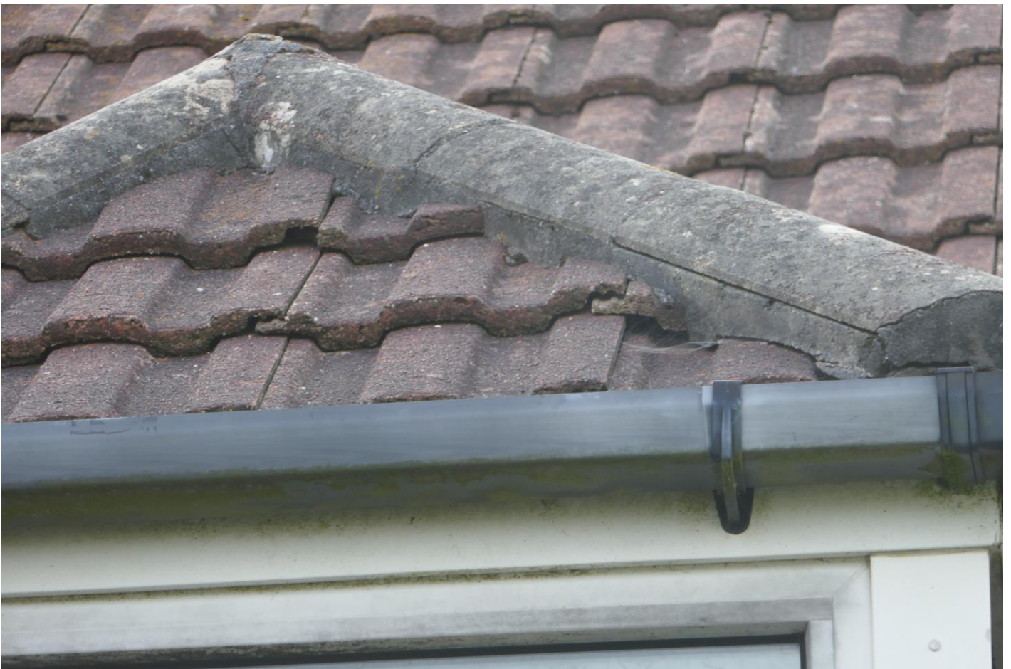
Figure 4. Gaps beneath roof tiles.
