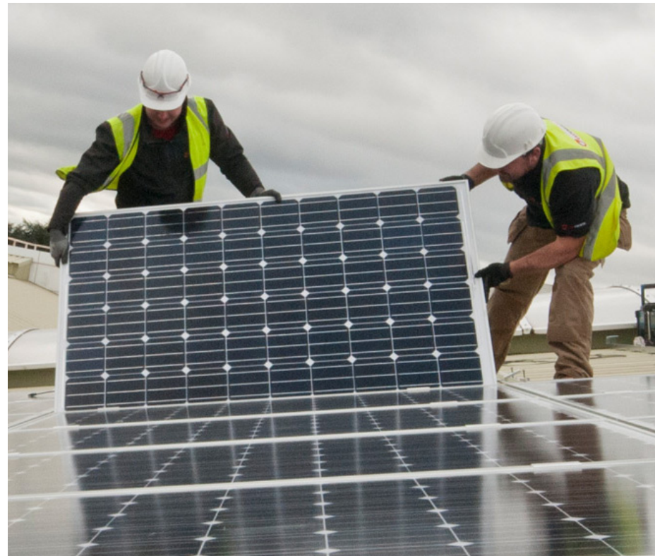
A PV array will be installed at roof level
