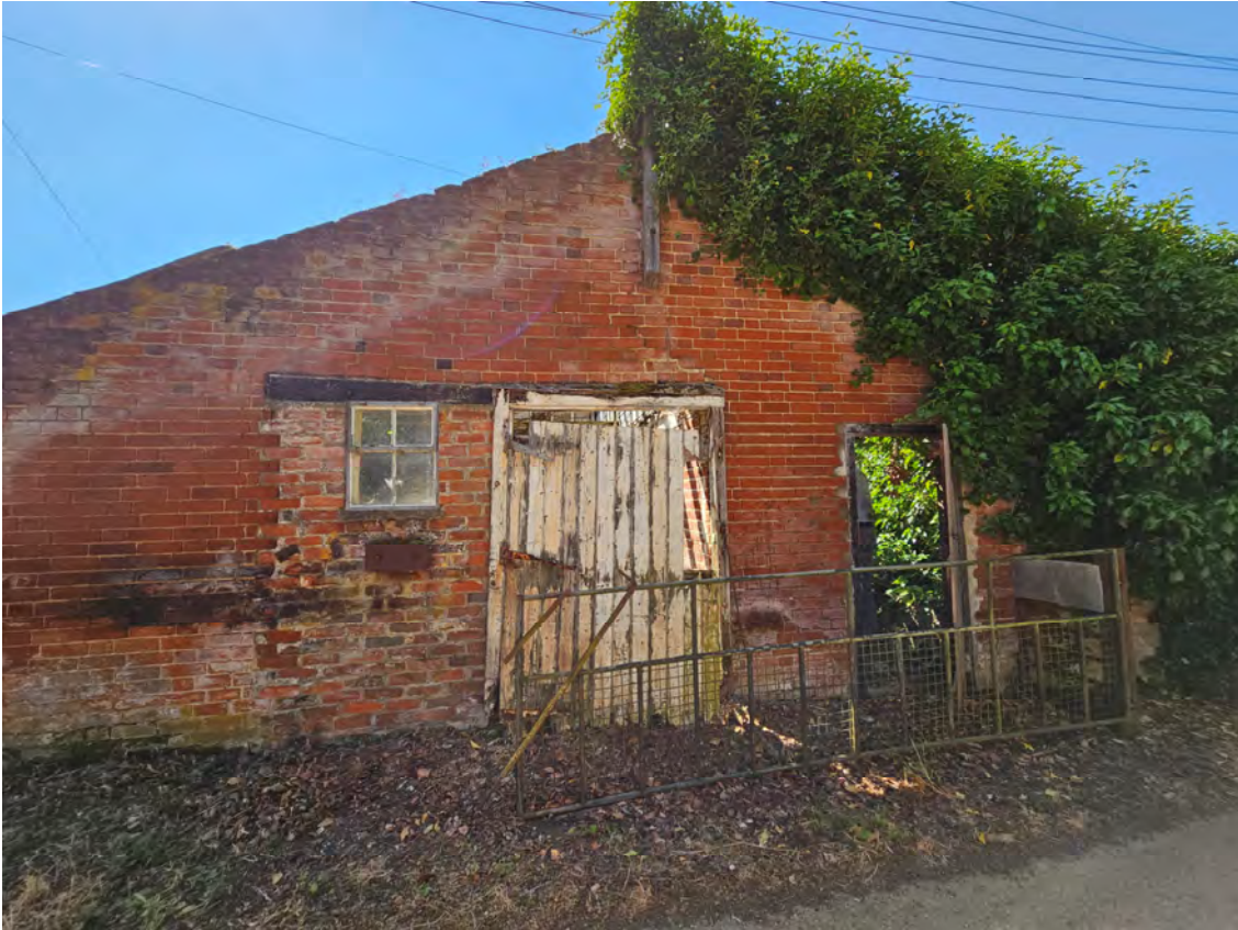
Photograph 2 : Dilapidated brick building on the south side of the track on the east side.
