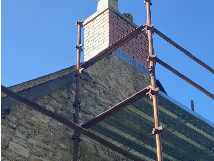
North gable end with remaining render at apex
