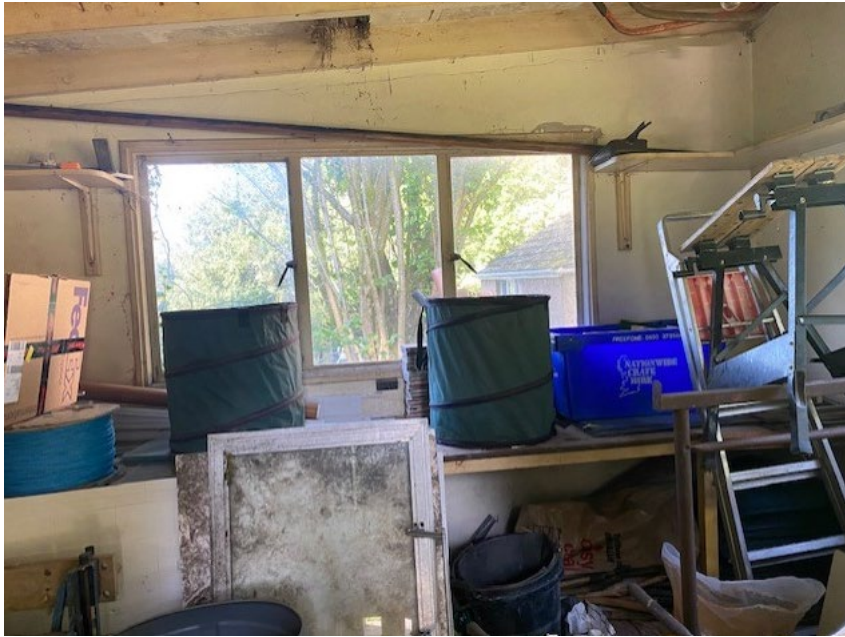
Interior of store room – north end of outbuilding – well used and with no ‘fly-in’ access
