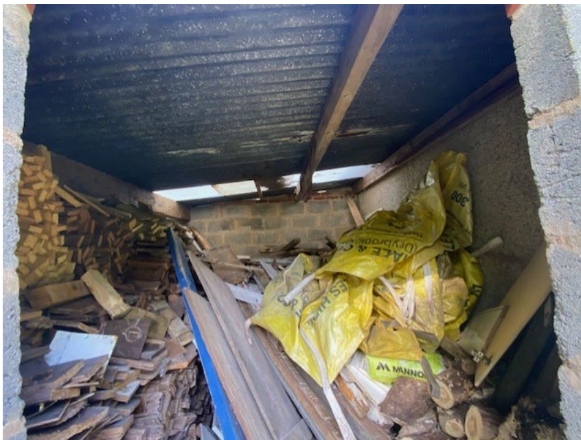
Interior of shed south end of outbuilding – high light levels and disturbance with absence of suitable likely perching locations and sufficient clearance reducing potential for bat or nesting bird use
