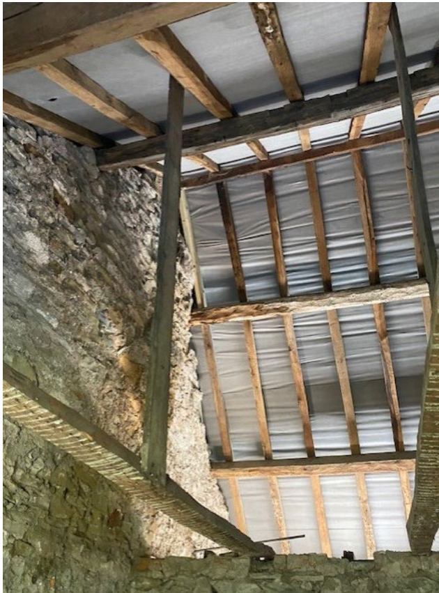
Inside first floor of house looking through removed ceiling area to exposed roof
