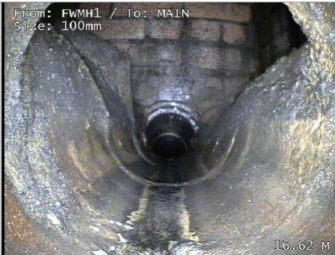
Finish node type, manhole, reference FWMH2
