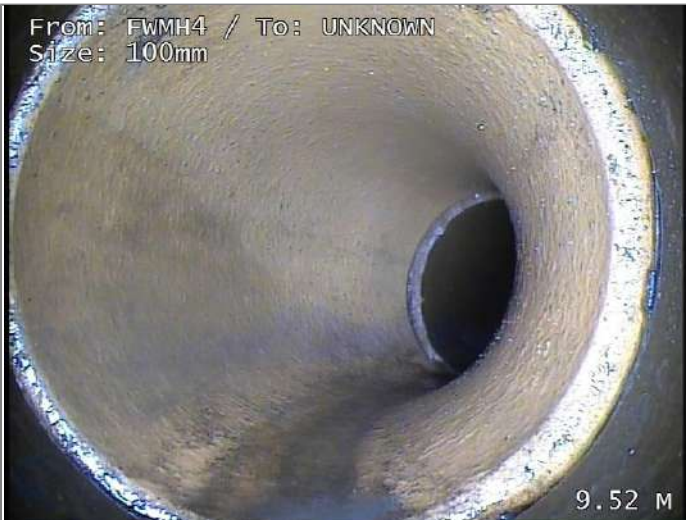
Line of drain/sewer deviates right
