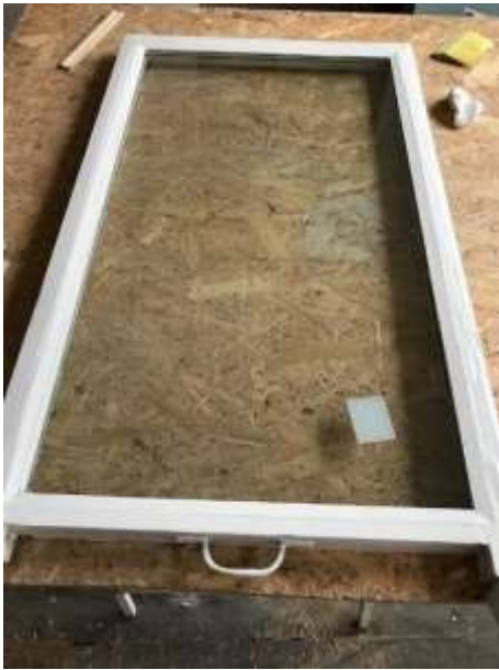
3. Double glazed unit installed into the existing sash – a look at the external glazing bead
