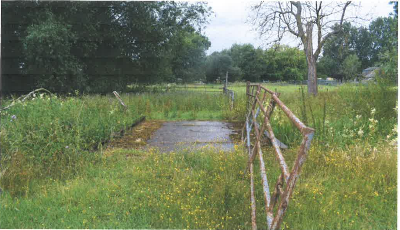
Concrete and steel agricultural bridge at the north of Time Out Farm
