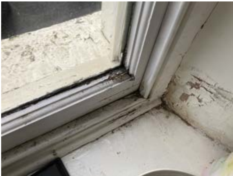
Photograph 10 – Typical internal view of sash window. Note the poor condition of the frame.
