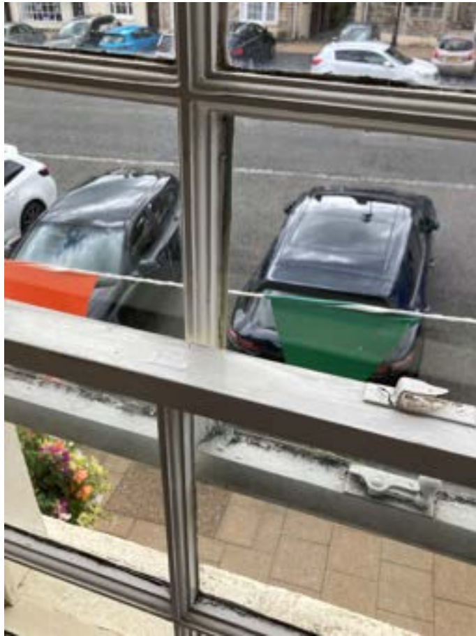
Photograph 09 – Internal view of sash window. Note the poor condition of the frame and glazing bars.
