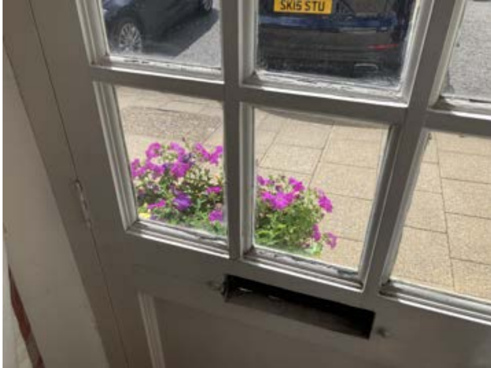
Photograph 07 – Typical internal view of the door to which this application relates. Note the state of disrepair.
