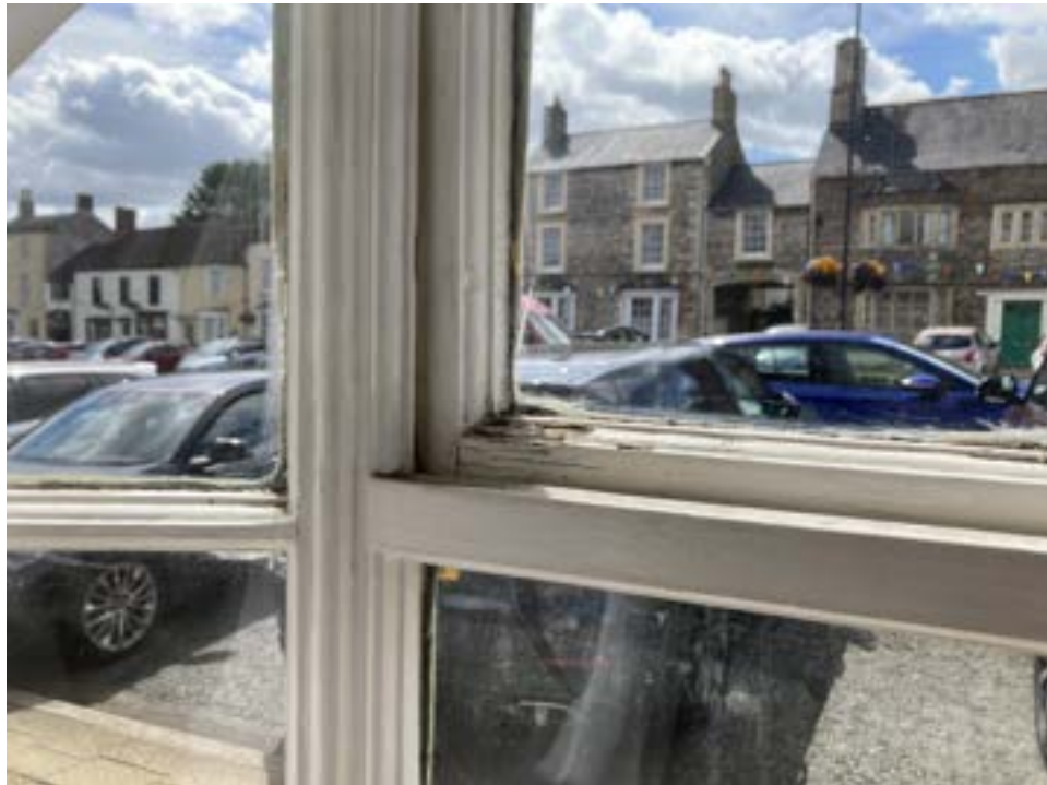
Photograph 05 – Typical example of poor condition of bay window frame.
