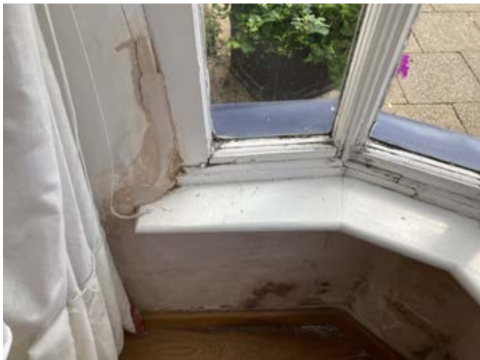
Photograph 06 – Typical internal view of bay window. Again, note the damp issues and poor condition of softwood joinery.
