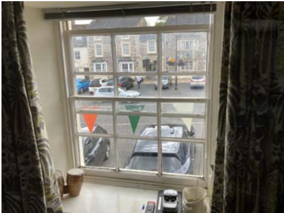
Photograph 08 – Internal view of first floor sash window to which this application relates.
