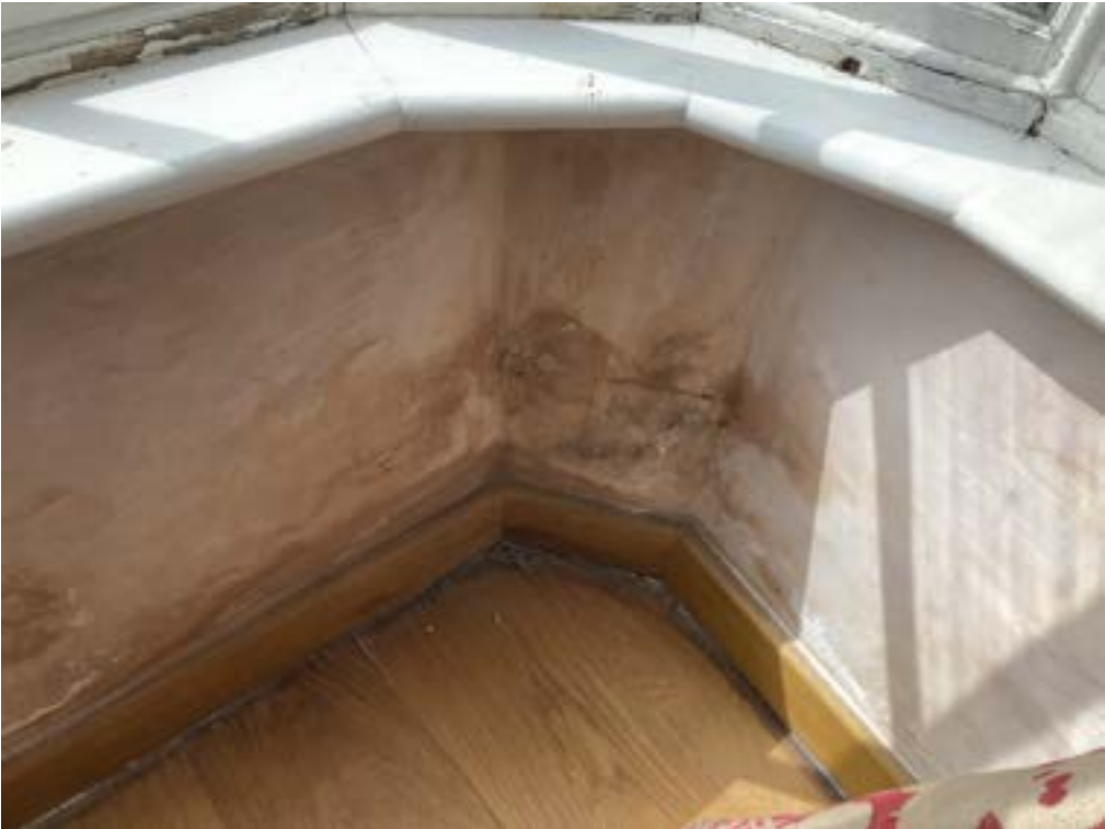
Photograph 04 – Internal view of the bay window plinth wall. Note the damp issues.
