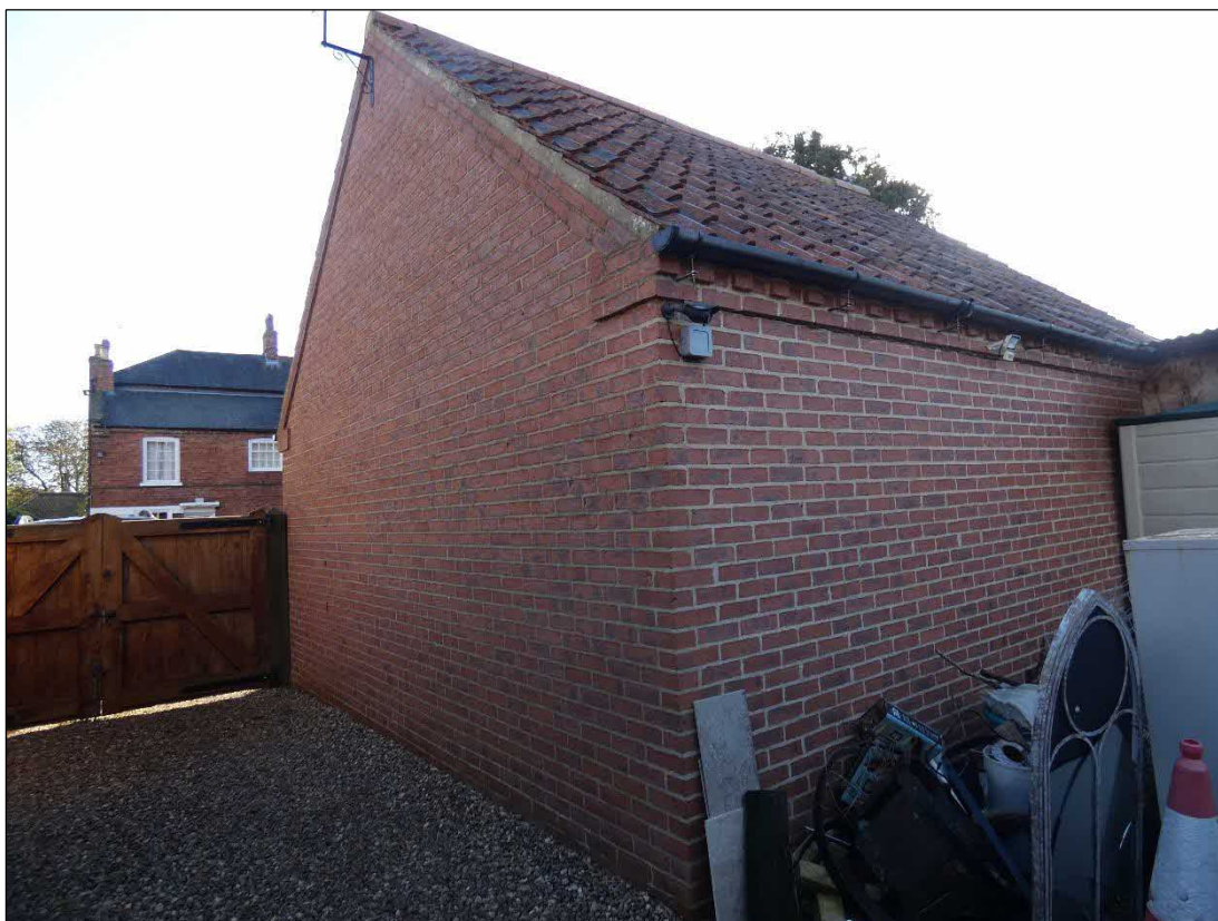
Photograph 1.3.4 : View of the north and west elevations of Building 3 (the garage) from its north-west corner.
