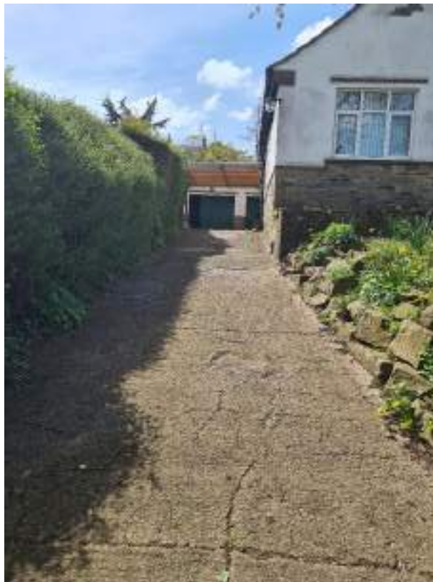
Photograph 2: A view of the rising driveway along the eastern side of the site. Note cracked, but otherwise good quality concrete.
