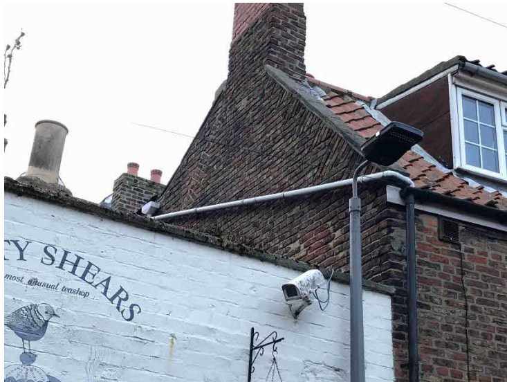
Photo 2 South gable, raised brick to rear with original 'brick tumbling' below copings
