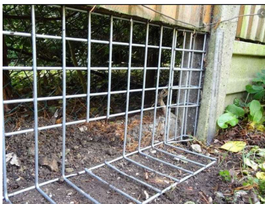
Insert 5: Showing wildlife access gap within fencing.
