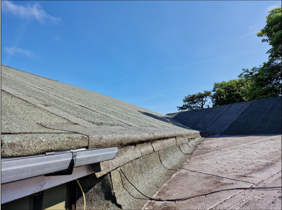
Plate 7 – General character of the bitumen 1F lining on the roof of B1
