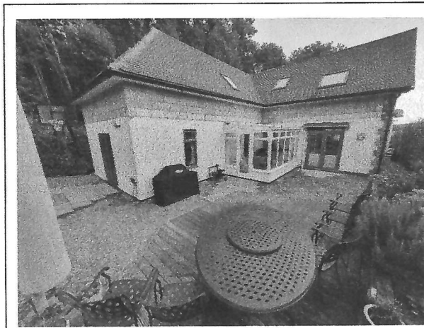
Fig 5: Site of the existing conservatory to be demolished and replaced with an extension.
