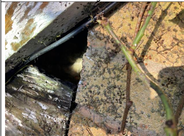
Photo 5 PRF at soffit southern corner
