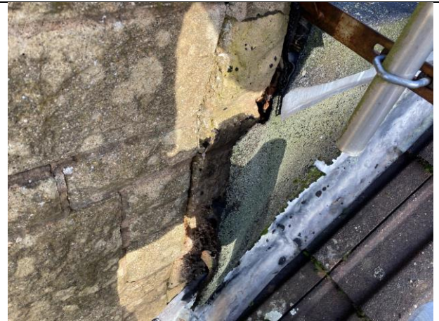
Photo 8 PRF behind felt at chimney
