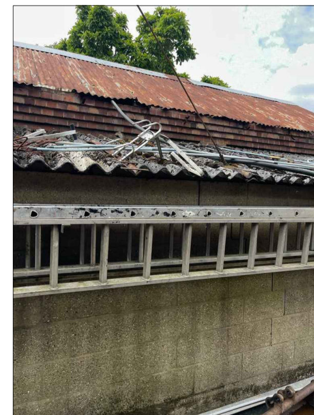
Side elevation of asbestos sheets on lean-to & rusting metal sheets to main roof pitches
