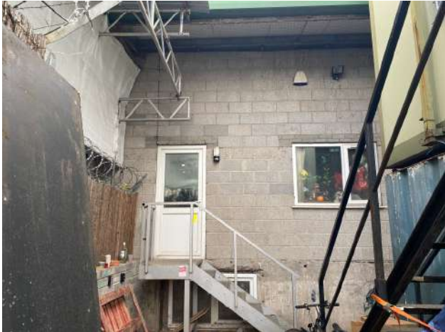
Plate 6: Crack in wall of east face B2 to left and above door
