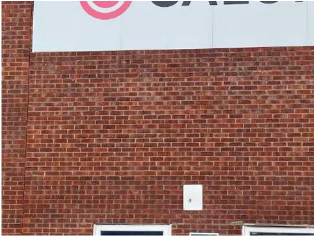
Plate 4: Crack in the Calor Gas buiding west face
