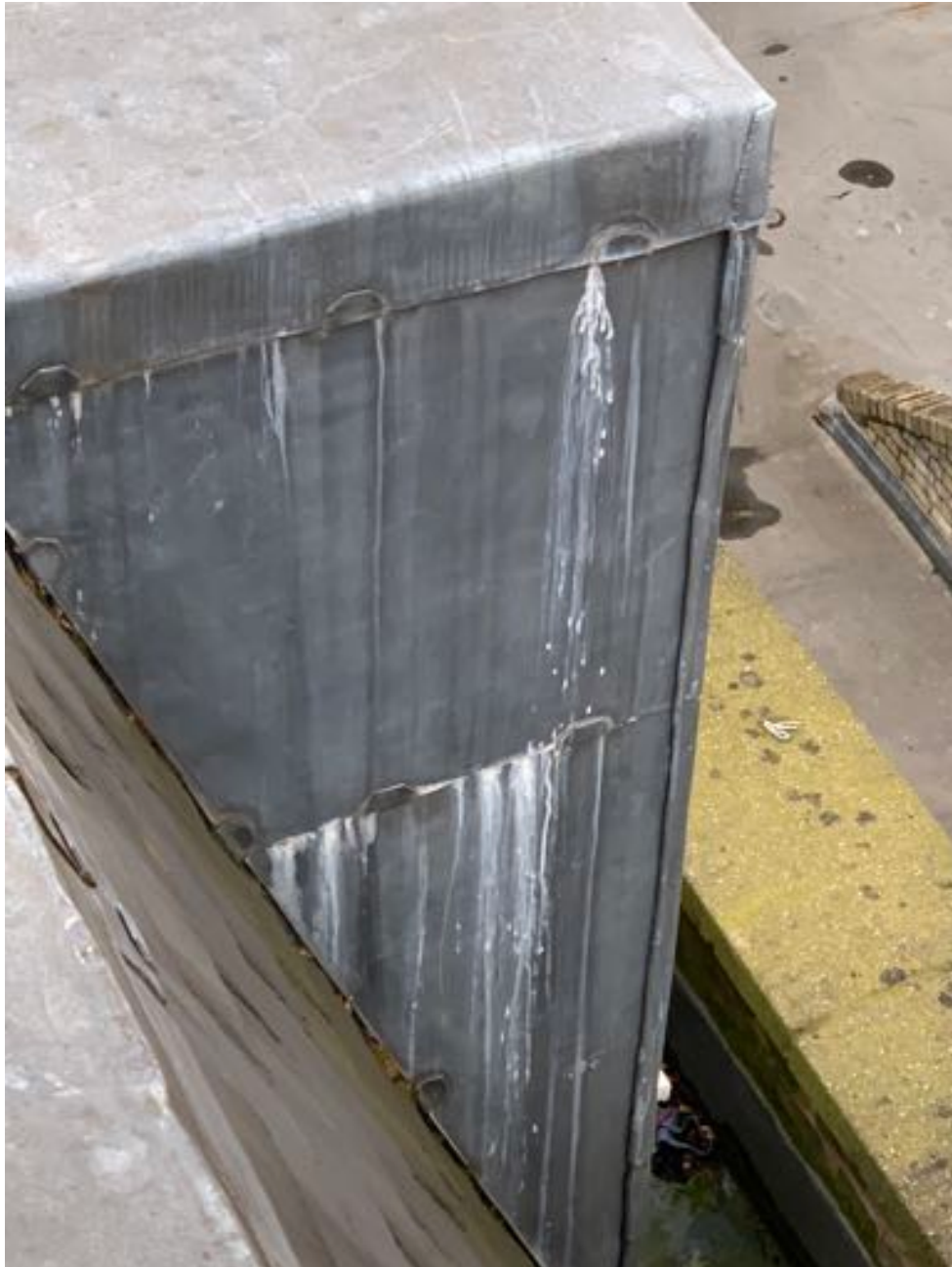
Photo E : Lead hydroxide formation to the existing roof dormer due to the lack of natural air ventilation
