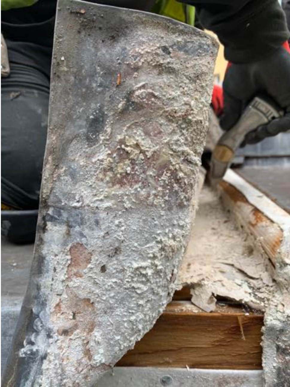
Photo D : Corrosion to the underside of the lead roof due to the lack of natural air ventilation
