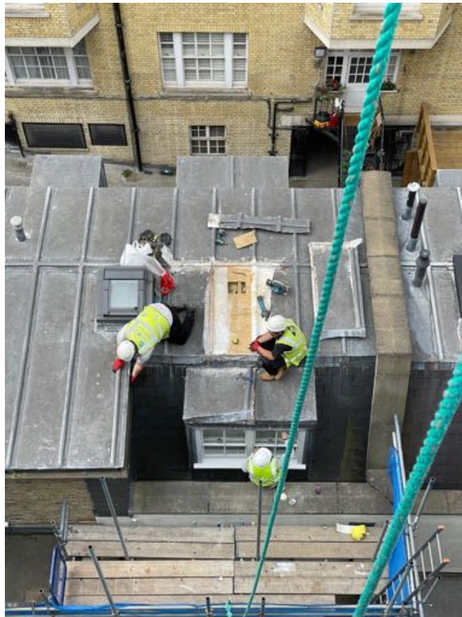
Photo C : Roof to the mews property at the rear of 57 Great Cumberland Place
