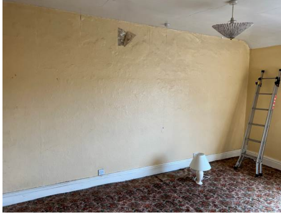
Damp external wall Bed 2
