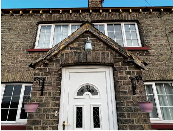
Front of house with decayed timber
