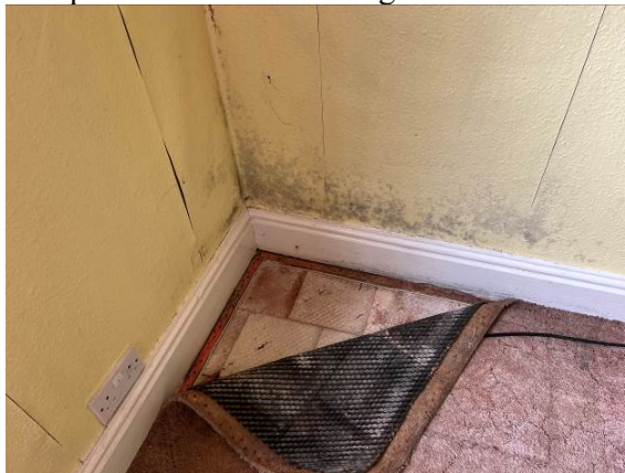
Damp floor and walls Dining Room
