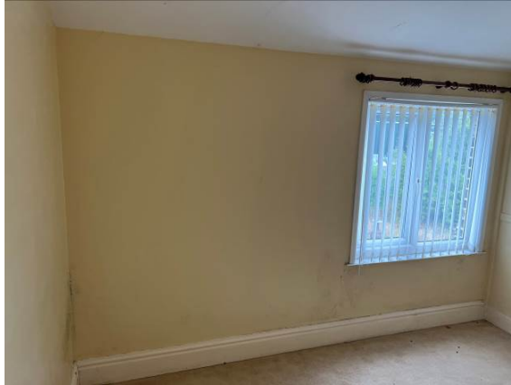
Damp external wall Bed 3
