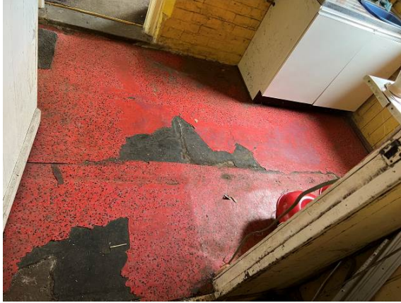
Damp Kitchen Floor
