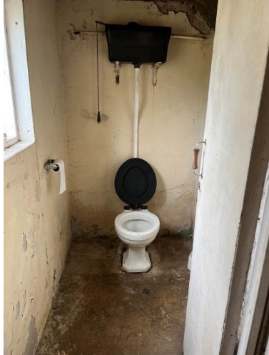
Damp walls, floor and ceiling GF WC
