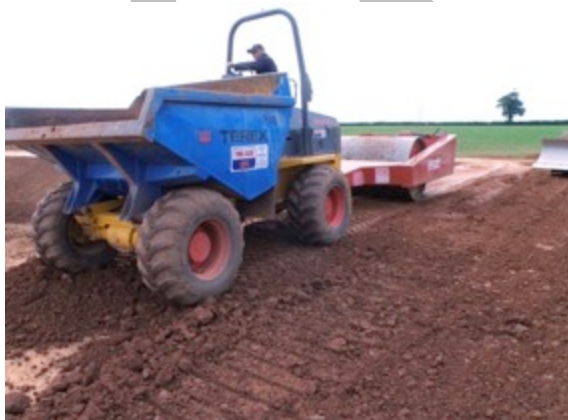
A shallow (100-150mm) layer of soil with 20-30% clay content is being laid up and rolled 4-6 times by a heavy vibrating roller to ensure adequate compaction
