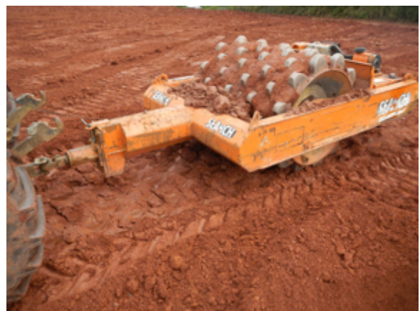
Here, a shallow (250 mm) layer of soil with 30-40% clay content is being rolled 4 times by a 2 metre wide 8 tonne vibrating roller to ensure adequate compaction
