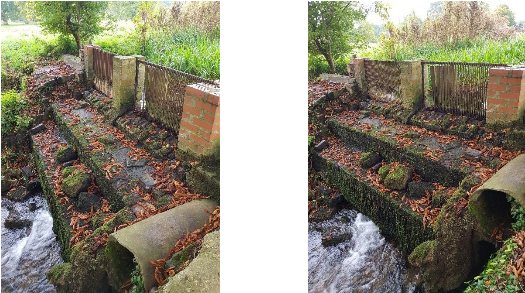
Figure 22 Looking southwest across the front of the weir with concrete sluice pipe on north bank.
