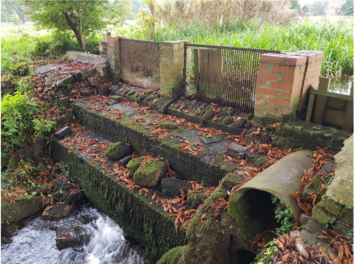
Figure 18 Looking southwest to the east side of the weir with the lake behind.
