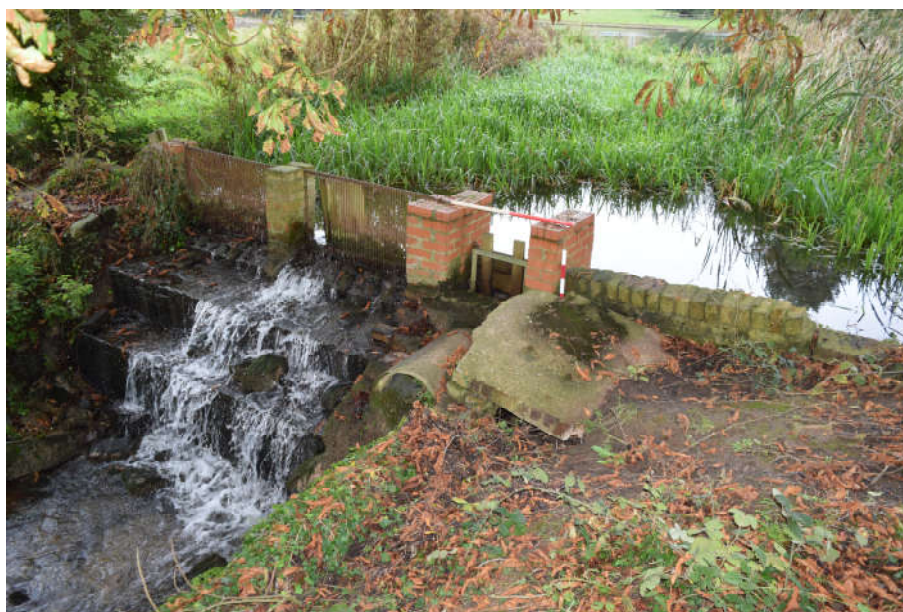
Plate 1: View of the weir, looking southwest. Scales are 1m and 0.4m (the latter is partially hidden)
