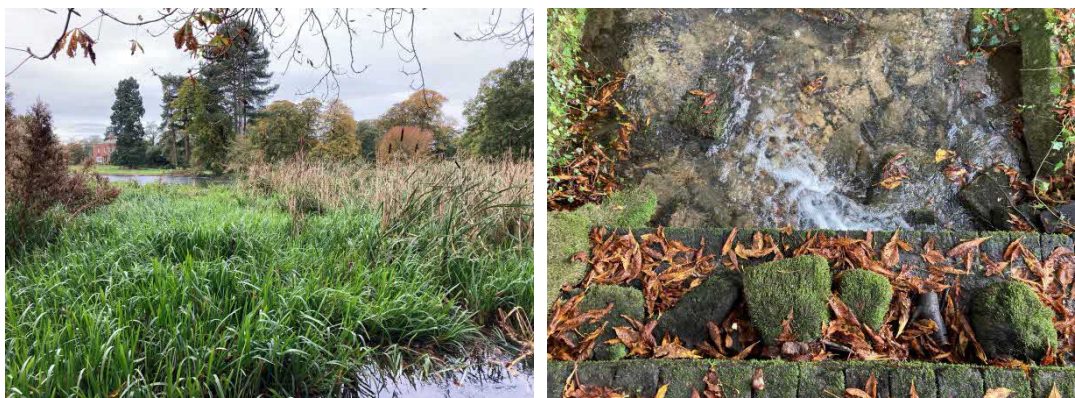
Photograph 3: Representative images of silt bed to the west of the weir (left) and eastern 'foot' of the weir (right).
