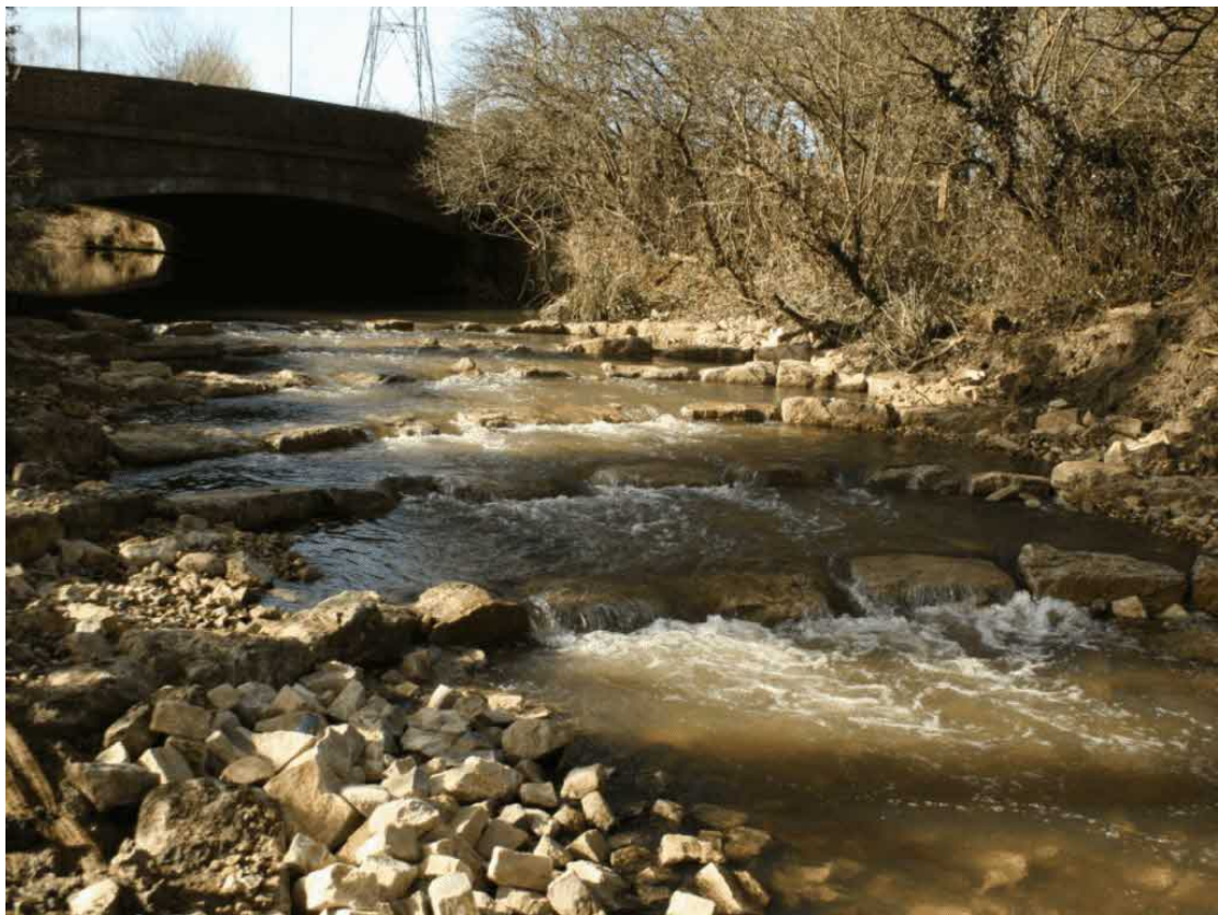
Fig 18. Before (above) and after (below) images of A240 weir removal, Hogsmill River, Surrey. Rock ramps were used in multiple locations to reconnect the chalk stream as part of the Hogsmill Connectivity Project.
