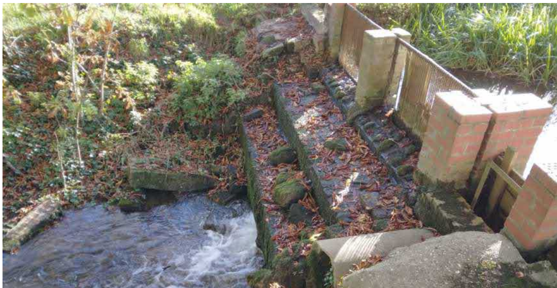
Fig 13. Existing weir, November 2023, highlighting water passing underneath the weir
