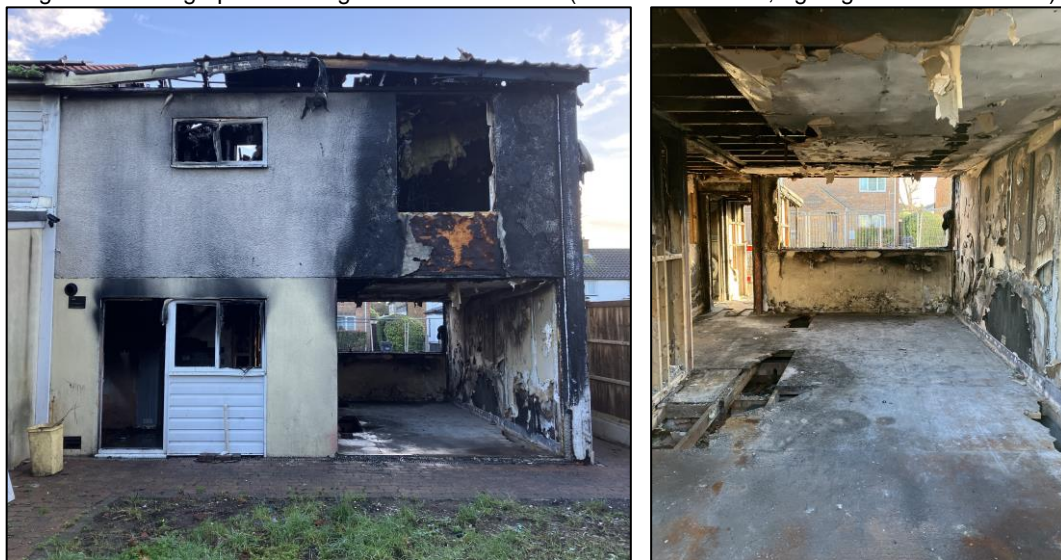
Figure 2: Photographs showing current state of site (left: rear elevation; right: ground floor interior)
