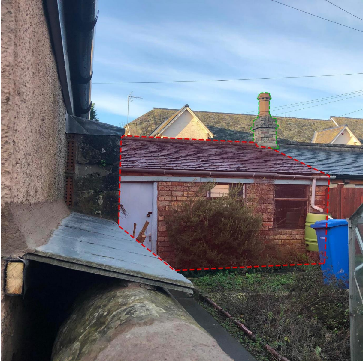
Figure 2. Front elevation of existing outbuilding as viewed from access pend. Portion to be demolished highlighted in red, shared chimney to be retained highlighted in green.
