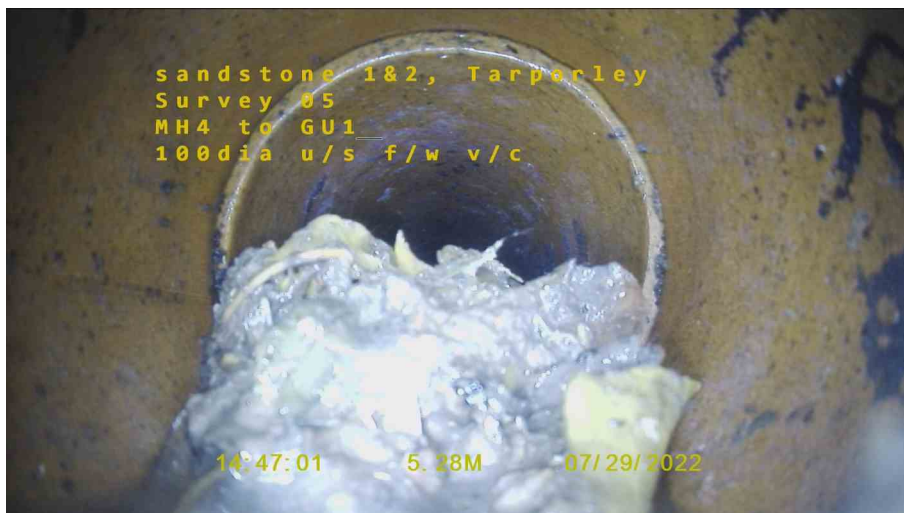
GU1X_2e384199-7d52-425a-81c6-0adef25e5c91_20220729_162546_858.jpg, 00:00:45, 5.08 m Settled deposits, coarse, 35% cross-sectional area loss
