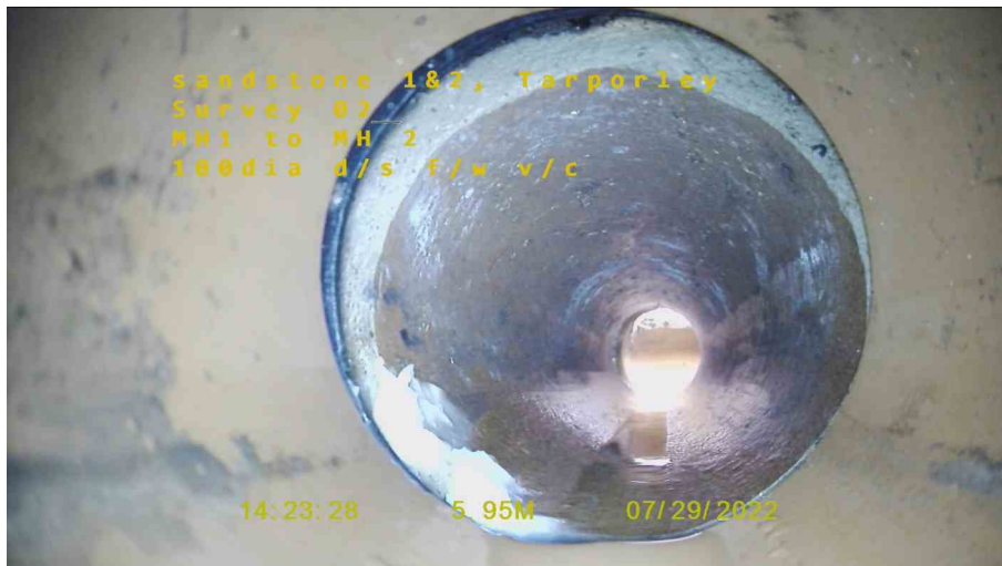
MH 1X_0023ac56-a4f5-4e78-a38b-39d076f0cd99_20220729_161027_832.jpg, 00:01:08, 5.95 m Joint displaced, medium
