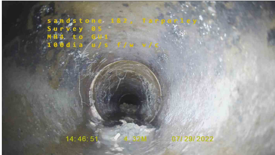
GU1X_159935f1-e943-4bbf-917c-08b571e269dc_20220729_162028_195.jpg, 00:00:37, 4.32 m Settled deposits, fine, 15% cross-sectional area loss
