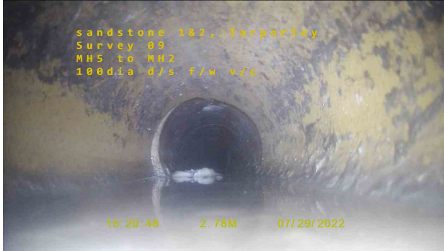
MH 5X_ab7737c4-07ad-46a8-9165-6def9d88c074_20220729_165107_540.jpg, 00:01:07, 2.78 m Joint displaced, medium
