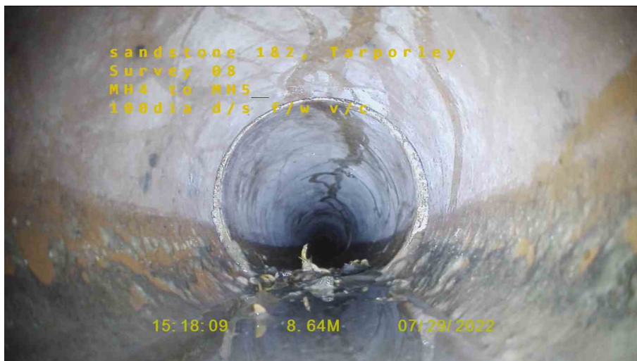
MH 4X_f9567e28-1b8f-4a3b-948b-f87abbf7b12a_20220729_163710_765.jpg, 00:01:00, 8.64 m Joint displaced, medium
