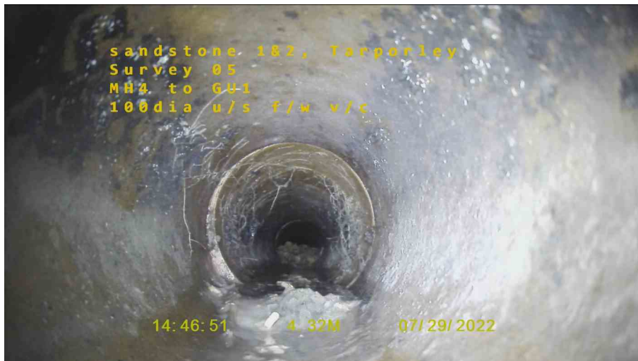
GU1X_337aec0a-ce45-4485-b1ab-c49e8cc39dd0_20220729_162038_416.jpg, 00:00:37, 4.32 m Joint displaced, medium
