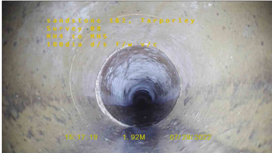
MH 4X_c45fb9b0-7eb8-4a4e-912a-c2cd59281794_20220729_163609_708.jpg, 00:00:13, 1.92 m Joint displaced, medium
