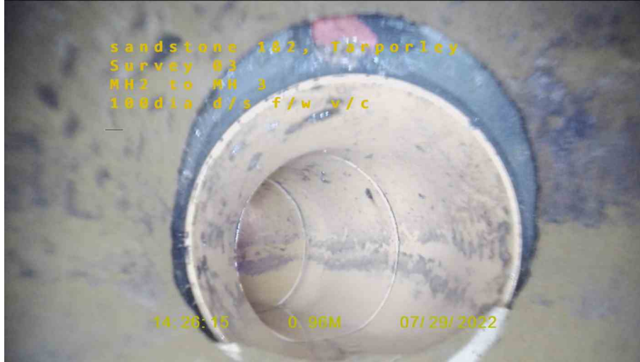
MH 2X_ee084e23-5be9-4afd-8df4-13e92c44d8c0_20220729_161306_891.jpg, 00:00:17, 0.96 m Joint displaced, medium
