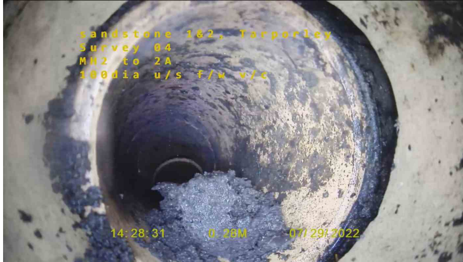
2AX_b9eef41d-b704-432d-9a8f-ce02de6b06b7_20220729_161632_476.jpg, 00:00:12, 0.28 m Joint displaced, medium
