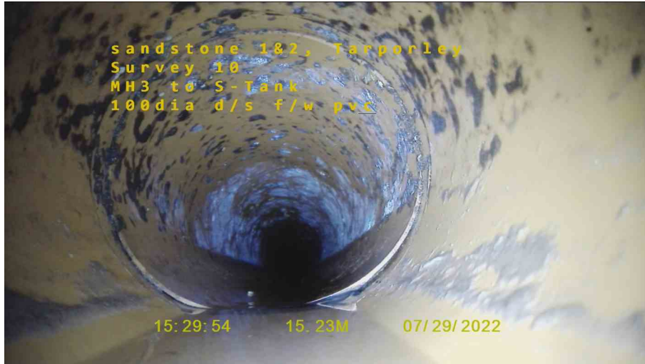
MH 3X_2cc578d8-d750-4956-a6d5-318fa0867966_20220729_170813_886.jpg, 00:01:38, 15.23 m Joint displaced, medium
