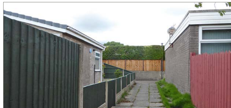
Blockwork wall, close board fencing and dense hedgerow / evergreen vegetation above the pedestrian access alongside Danbers. This will be retained post development
