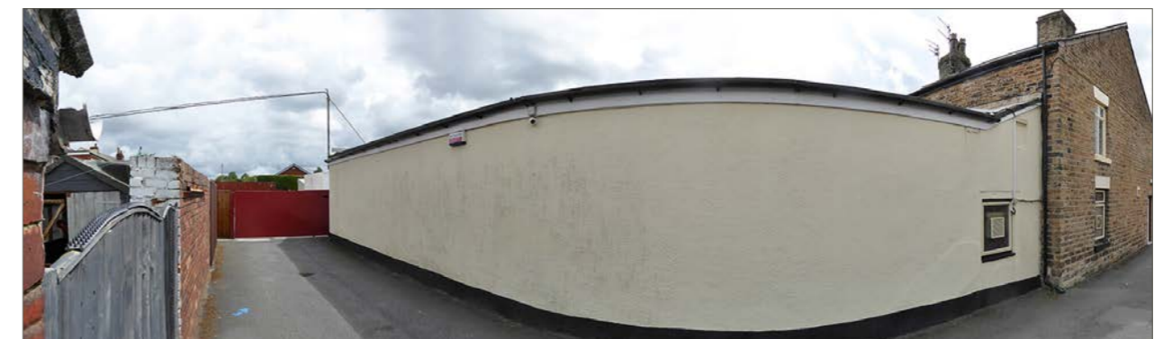
The existing north elevation. All rendered elements in the photograph are proposed shall be demolished to make way for circulation space, access and parking
