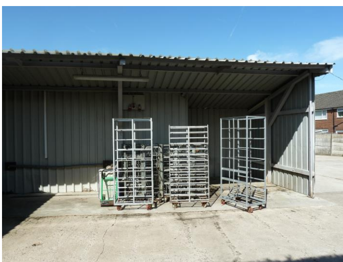
Photograph 21: - B2 general view of construction type of outdoor storage area. austere, single-skin, no gaps or void spaces.
