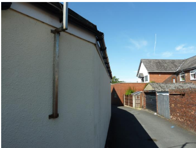
Photograph 16: - B2 the single storey flat-roofed building to the rear of B1. All fascia boards tight fitting, no gaps.
