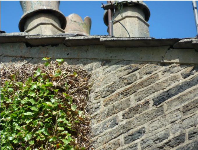
Photograph 4: – B1 mortar gap at verge – south gable elevation.
