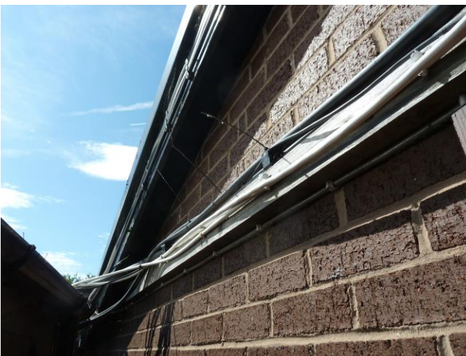
Photograph 30: - B3 rear elevation with soffit box fitted tight to wall. Steel verge capping over the top of soffit fascia has a gap but is unsuitable for roosting bats due to high temperature variations.
