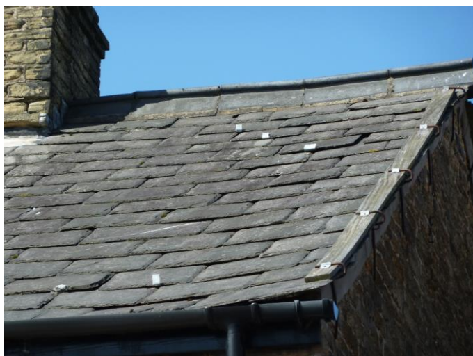
Photograph 15: – B1 roof rear elevation – several gaps below/between slates.
