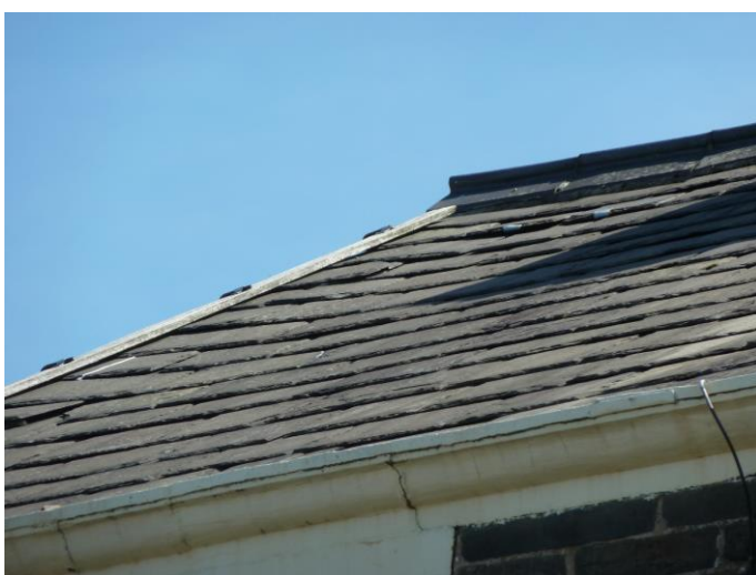
Photograph 9: – B1 gaps below slates – front elevation + small gap below batten (exposed).
