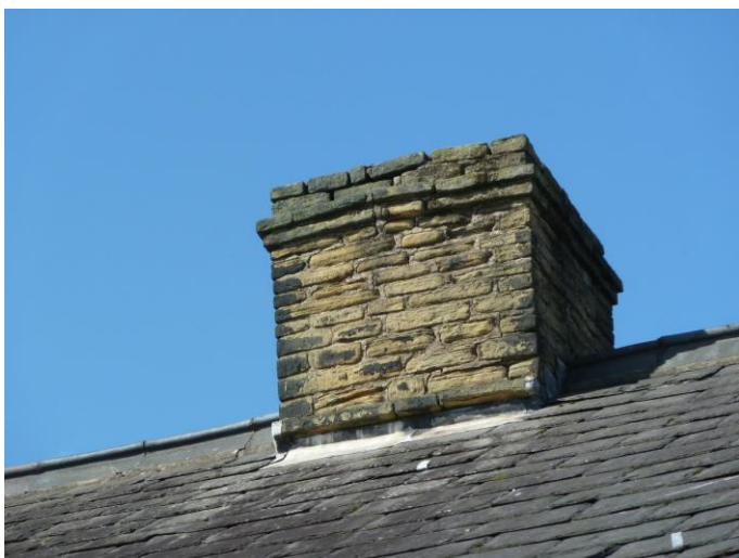
Photograph 11: - B1 chimney stack with mortar gaps along top course – probably subject to rain ingress.
