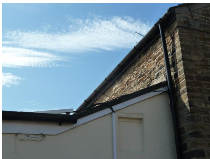
Photograph 13: – B1 gap behind fascia board east (rear) elevation – potentially leads to wall plate. The connecting rendered building is B2.
