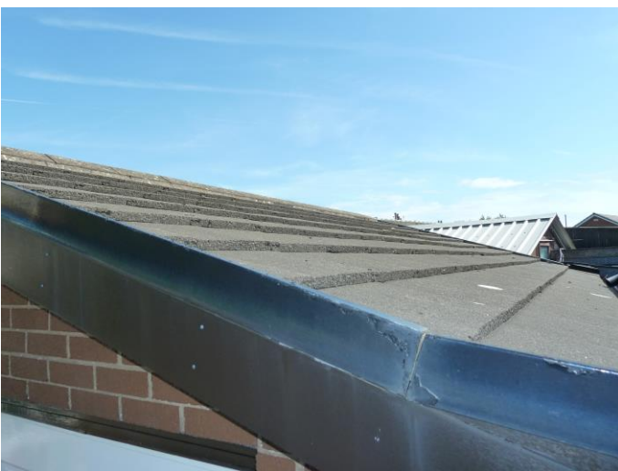
Photograph 34: - B3 front elevation with steel verge cap fixed to the wall and dry verge system above. Roof is in very good condition with no gaps.
