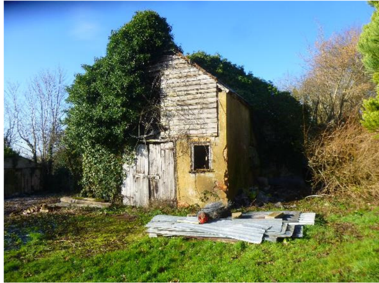
Fig.1.0 – Photograph looking towards existing building 3. As a result of the sites historical use, there is a large amount of paraphernalia littered throughout that give it a messy appearance.
