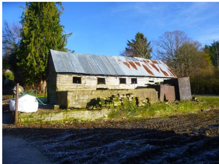
Fig.4.0 – Photograph showing existing building 11. The overall height of this building is further increased by the block retaining wall to the front. This elevation is to the south, which is perhaps the most visible part of the building.
