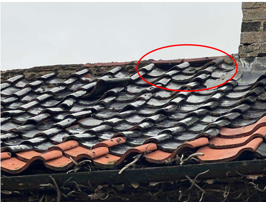
Photo 8. Building section 2 (ref B2A). Close up of roof as shown in photo 7. Shows missing mortar under ridge tiles as shown in red.
