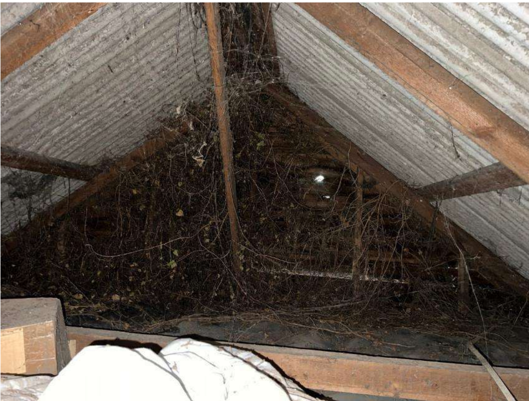
Photo 25. Building section 4 (ref B4). Internal view, looking towards southern gable. Shows dense ivy growth within roof space and exposed corrugated sheeted roof.
