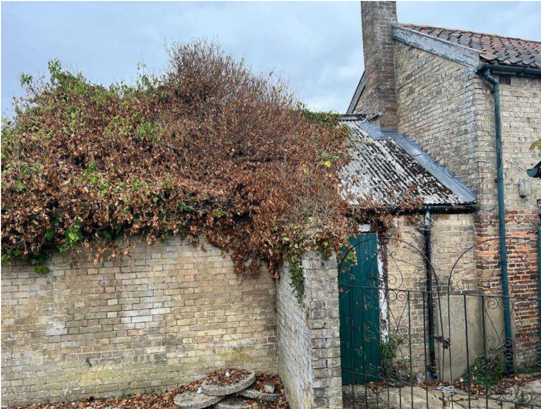
Photo 22. Building section 4 (ref B4). Shows section 4 adjoining section B3A. Most of the roof is covered in dense ivy growth (ref TN2).
