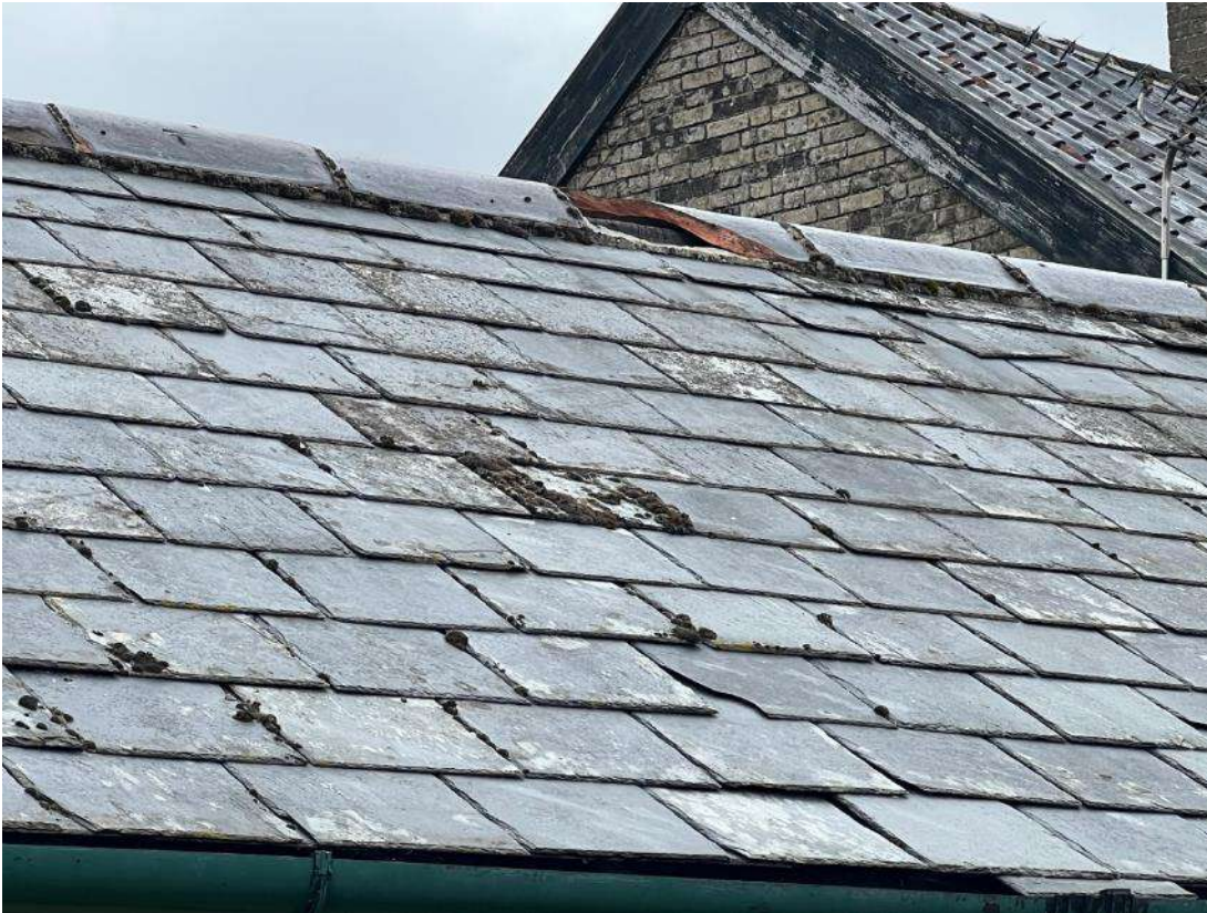
Photo 27. Building section 5. Shows close up of damaged ridge tile identified in photo 26.
