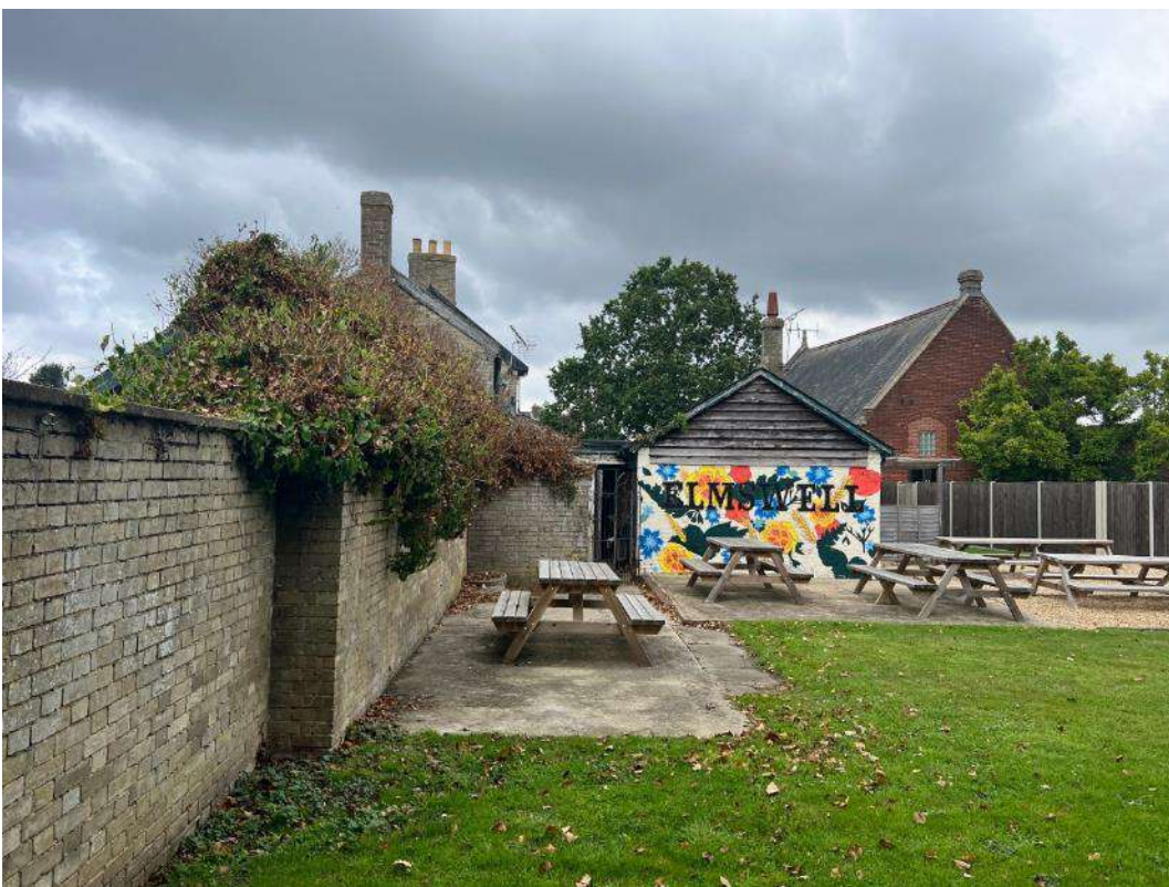
Photo 40. Taken alongside internal brick wall boundary to south of garden. Shows dense ivy growth at rear of section 4 (ref TN2).
