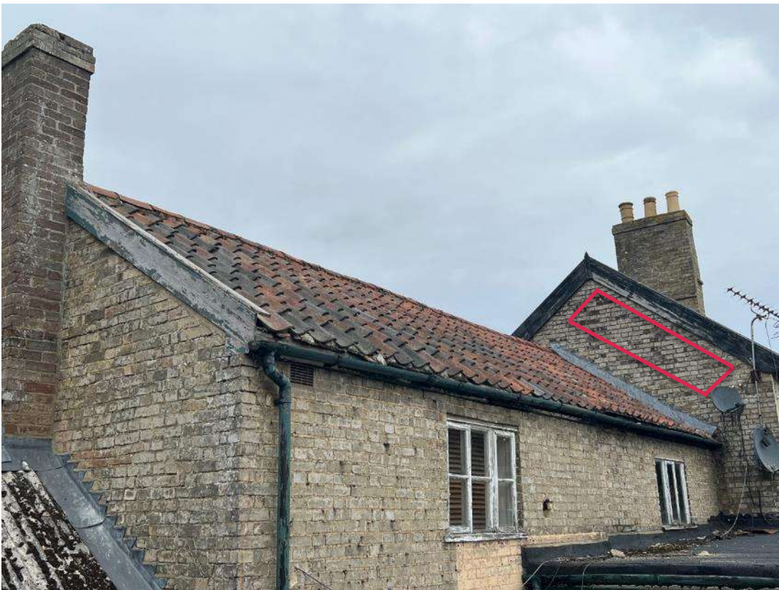
Photo 17. Building section 3 (ref B3A) adjoining section B2A. East aspect. Recommended location of bat boxes as outlined in red.
