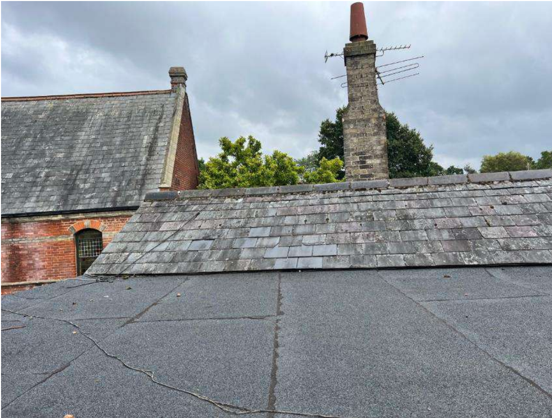
Photo 20. Building section 3 (ref B3B). Shows flat roof of section B3B adjoining section 5 (ref B5).
