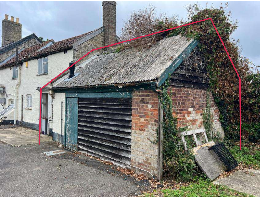
Photo 21. Building section 4 (ref B4). Outline of building shown in red. Shows western access point and timber cladding. There is a corrugated cement roof.
