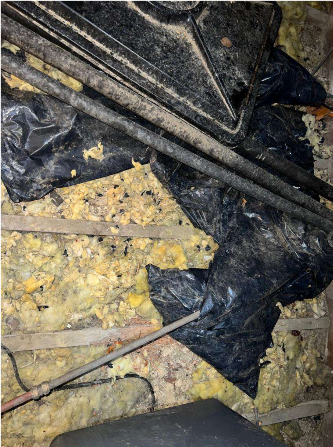
Photo 13. Building section 2 (ref B2A). Likely evidence of squirrel damage. A squirrel has been seen to enter the roof space of section 3 on multiple occasions during the survey visits.
