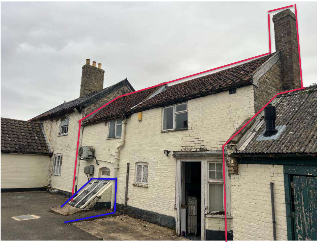
Photo 15. Building section 3 (ref B3A). West aspect of building. Extent of section 3 is outline in red. Cellar hatch and loading ramp is identified in blue.
