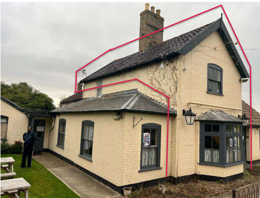
Photo 10. Building section 2 (ref B2A and B2B). Section B2A is outlined in red.
