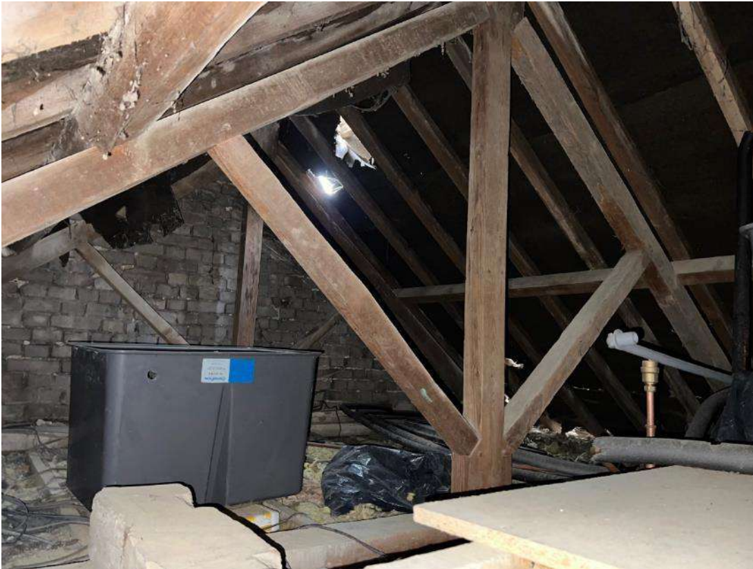
Photo 11. Building section 2 (ref B2A). Interval view of roof space. Shows damaged under felt and fire wall between section B2A and B3A. Taken from loft hatch.
