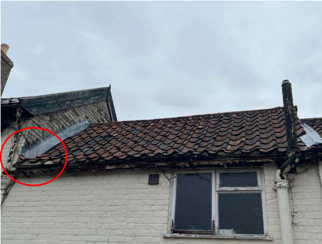
Photo 16. Building section 3 (ref B3A). Shows gap under lead flashing where section B3A adjoins section B2A as identified by red circle. Most of the gaps beneath the pan tiles are all mortar filled. West aspect.
