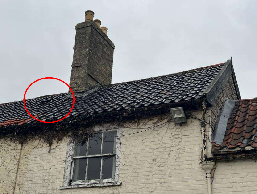
Photo 7. Building section 2 (ref B2A). Shows some slipped pan tiles as outlined in red. Evidence that this part of the building was covered with a climbing plant. This has caused damage to the fascia, soffit and under felt.
