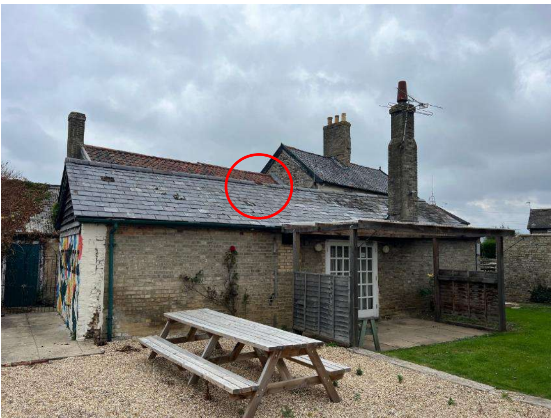
Photo 26. Building section 5. Shows eastern aspect of building along with pergola and patio area. Red circle outlines damaged ridge tile.
