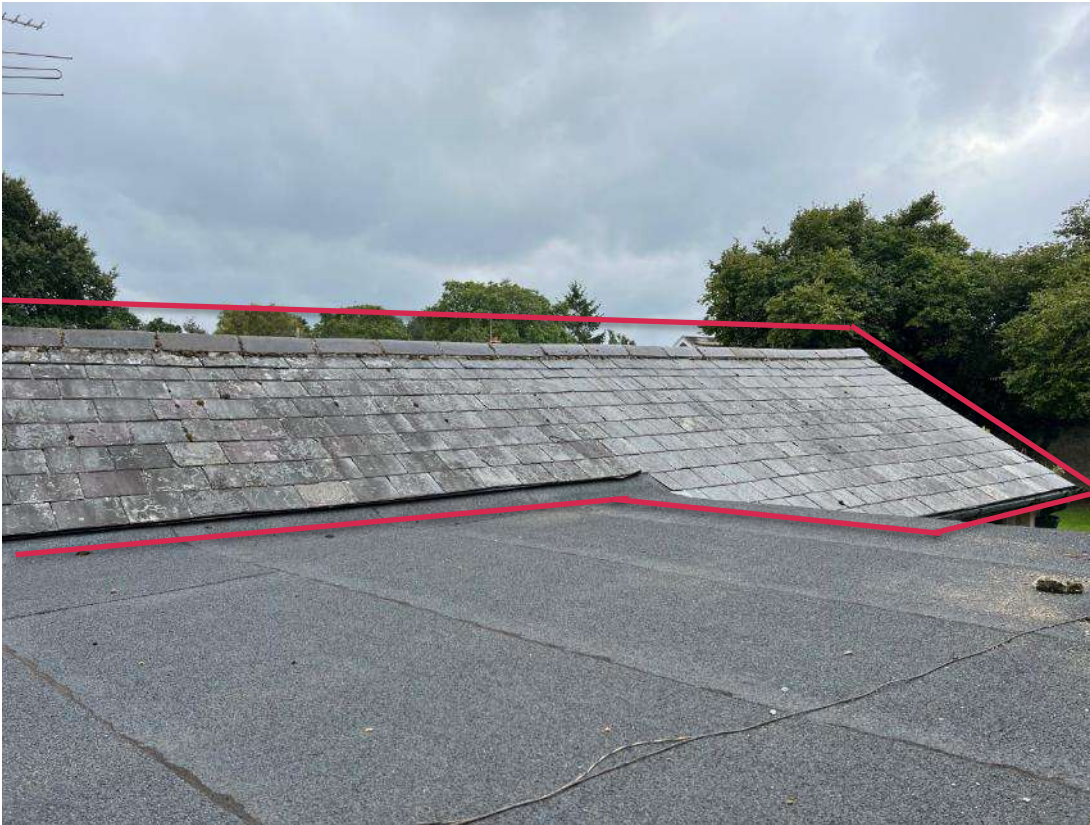
Photo 29. Building section 3 and section 5. Shows section 5 slated roof as outlined in red.
