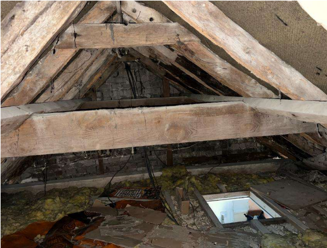
Photo 18. Building section 3 (ref B3A). Roof space. Shows old timber work and sarking underlay.
