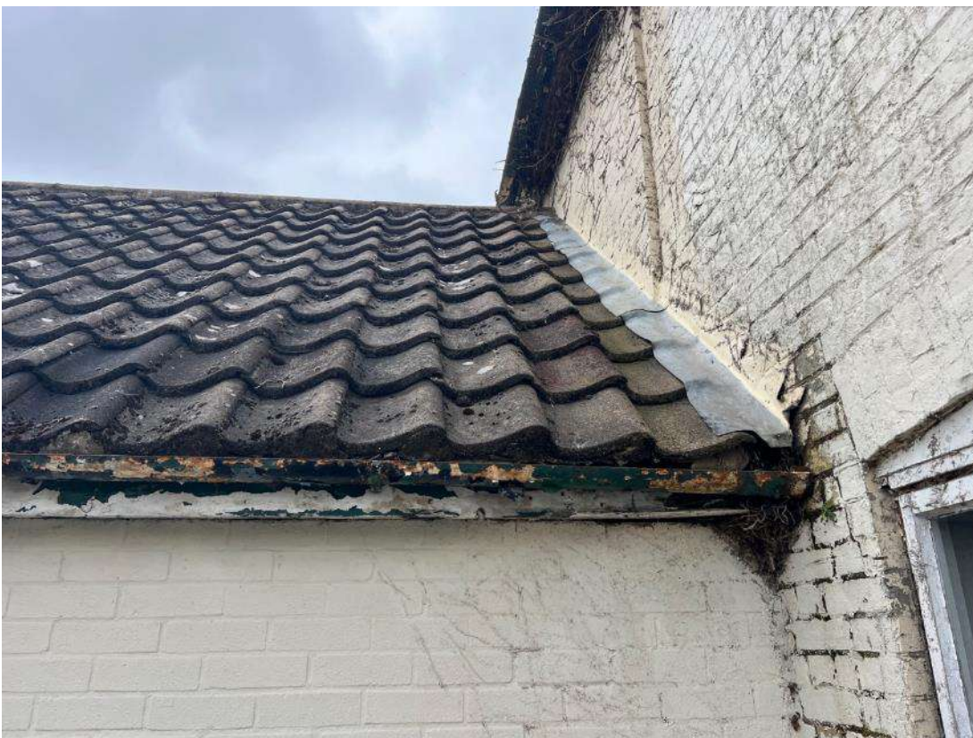
Photo 4. Interface between building section 1 and building section 2. Gap under lead flashing and damaged soffit/fascia. Evidence that this section of the building was recently covered in a climbing plant.
