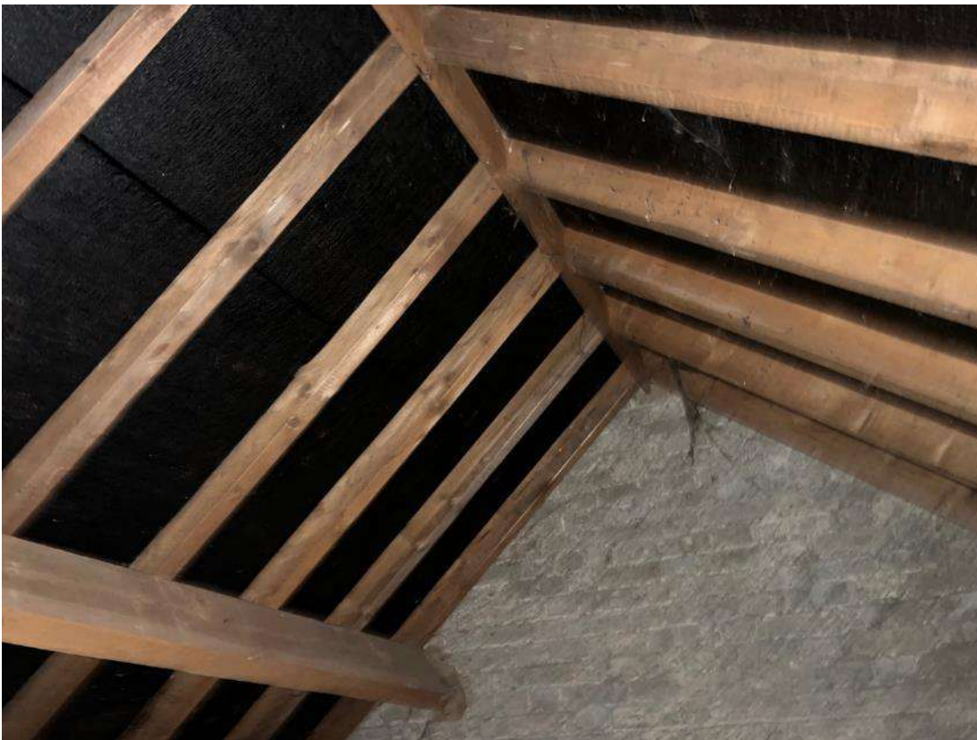
Photo 6. Building section 1. South end of roof space. No access points between building section 1 and section 2.
