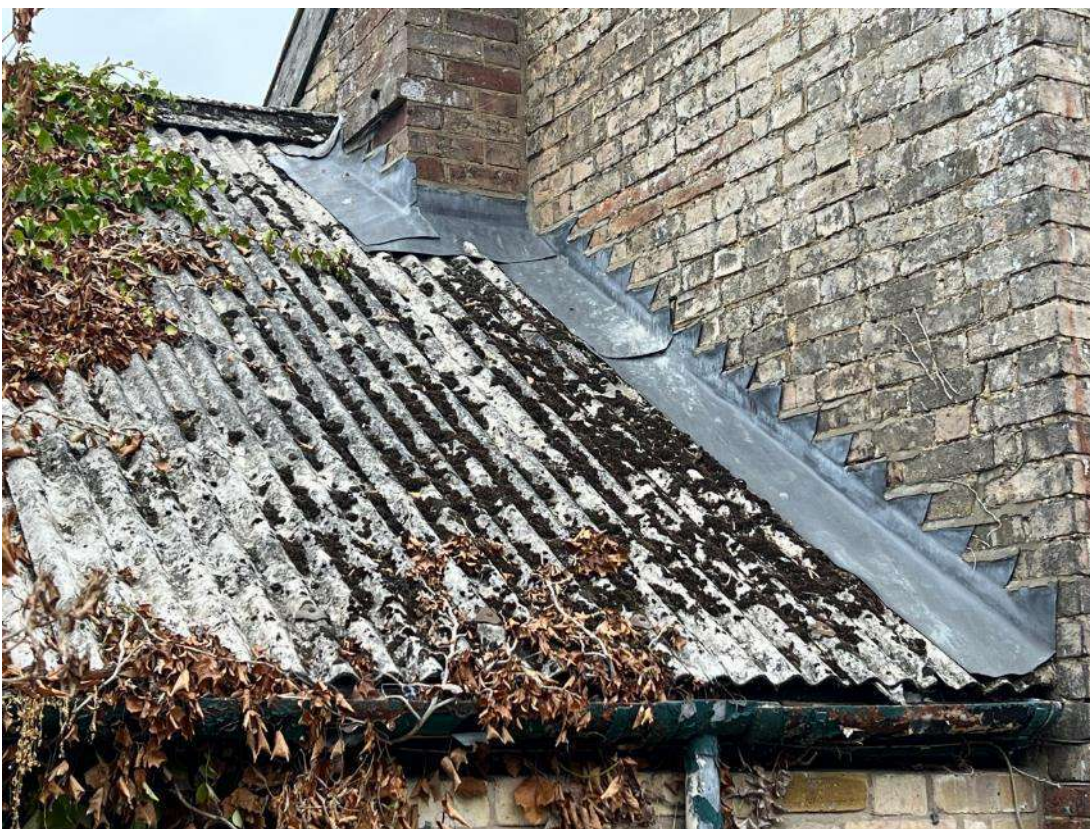
Photo 23. Building section 4 (ref B4). Shows gaps between roofing material and brick work. There are also gaps under corrugated ridge.
