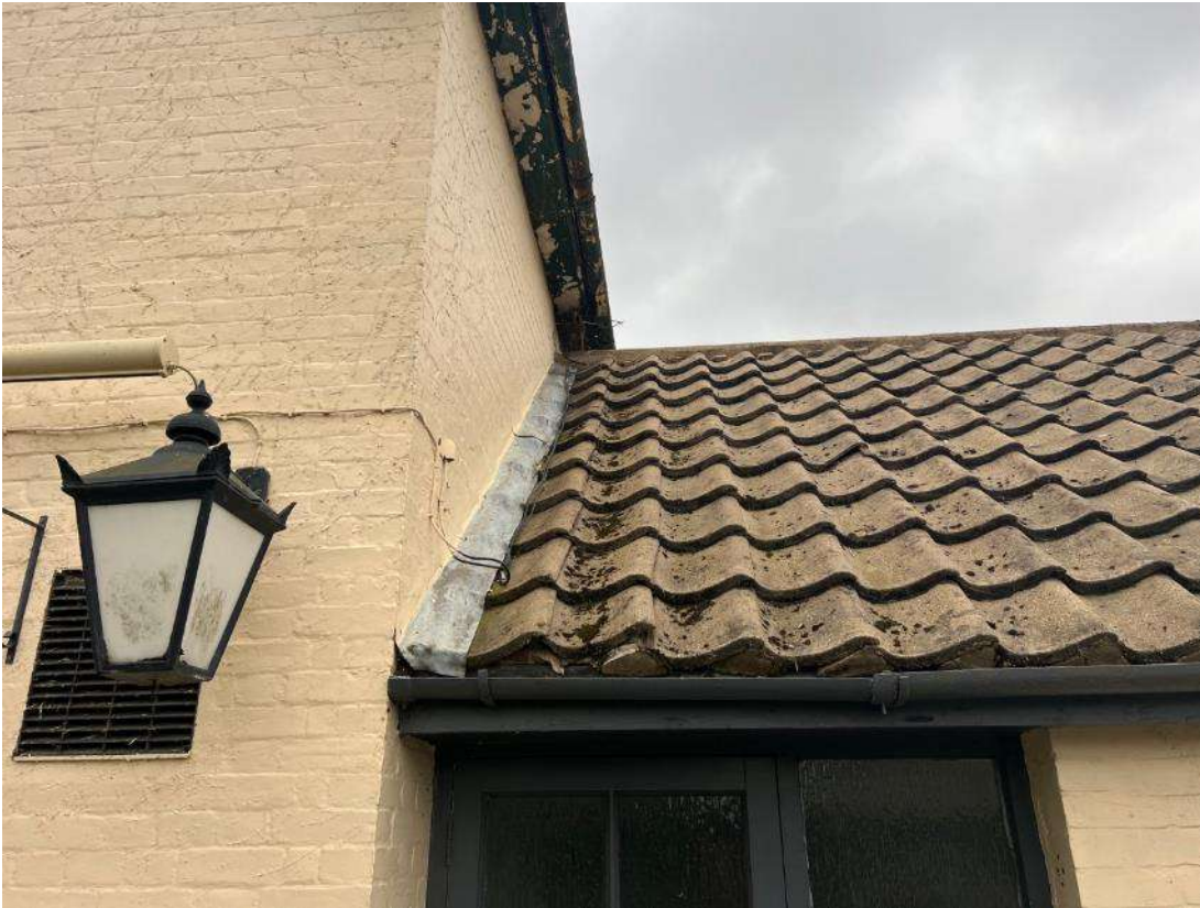
Photo 3. Interface between building section 1 and building section 2. Gap under lead flashing. Shows most of gaps under pantiles as being infilled with mortar. All gaps here, were cobwebbed.
