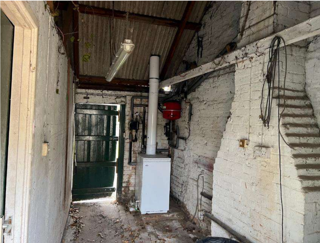
Photo 24. Building section 4 (ref B4). Internal view, looking towards western access point. Shows no underlay material.
