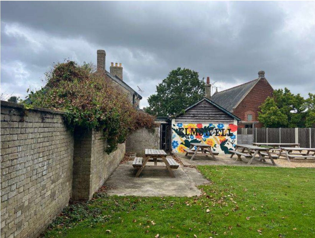
Photo 43. Taken alongside internal brick wall boundary to south of garden. Shows dense ivy growth at rear of building 4 (ref TN2).
