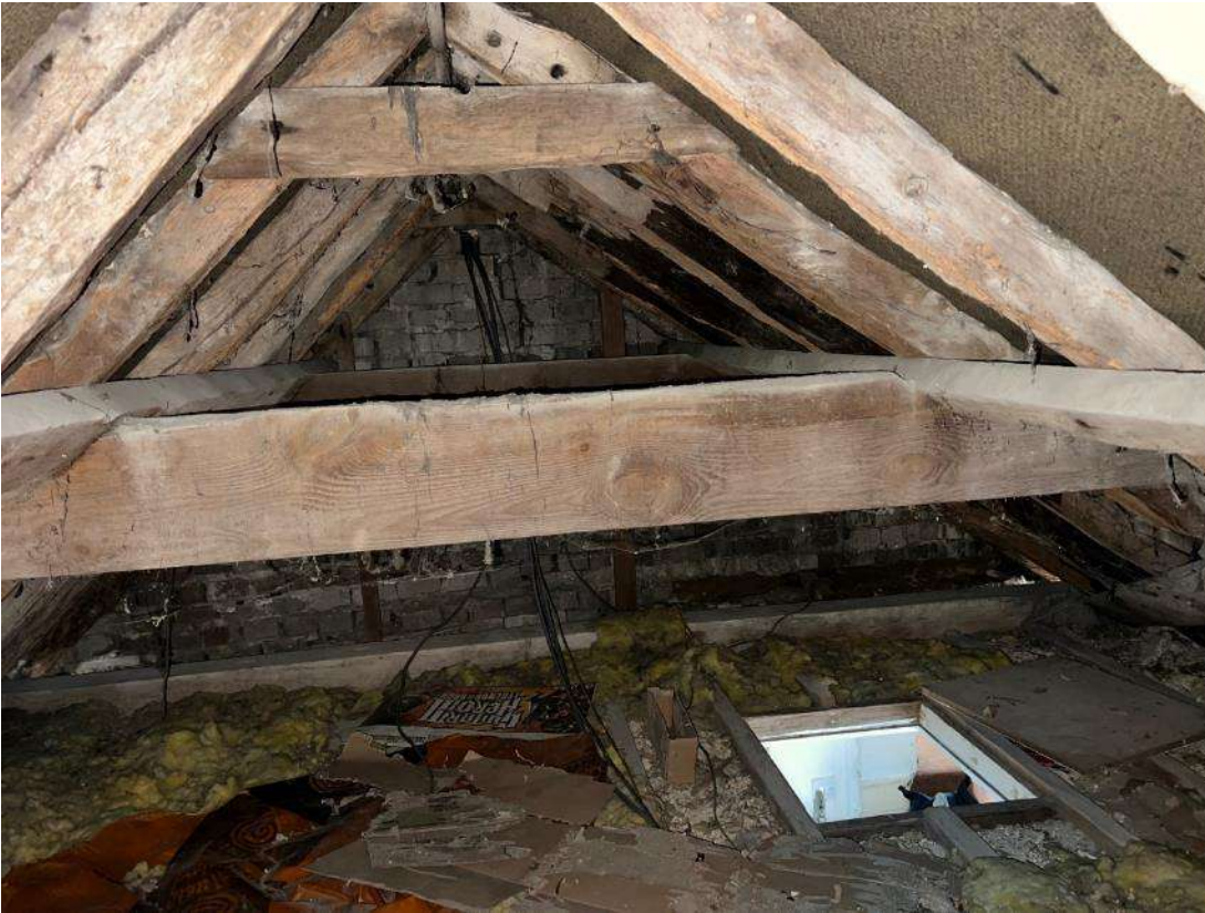
Photo 18. Building 3 (ref B3A). Roof space. Shows old timber work and sarking underlay.
