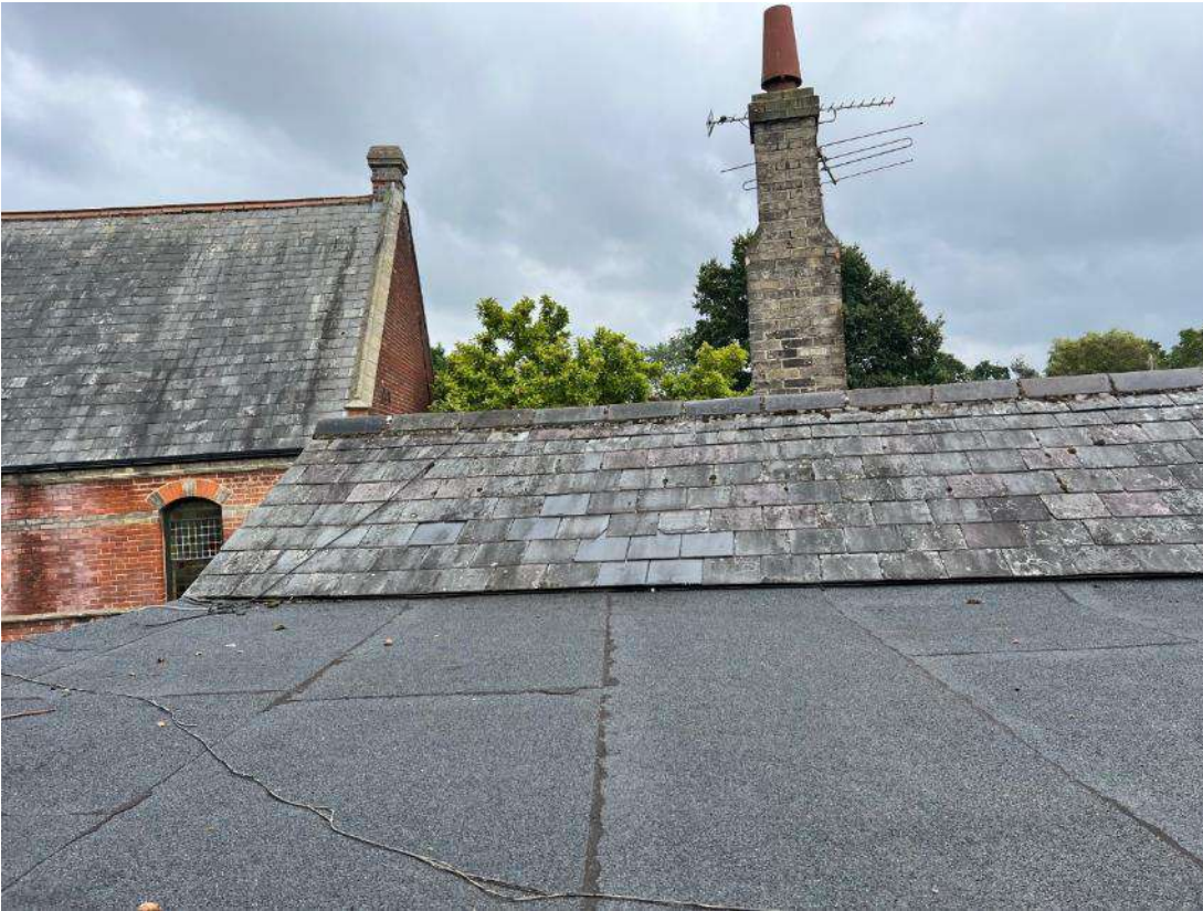
Photo 20. Building 3 (ref B3B). Shows flat roof of building B3B adjoining building 5 (ref B5).
