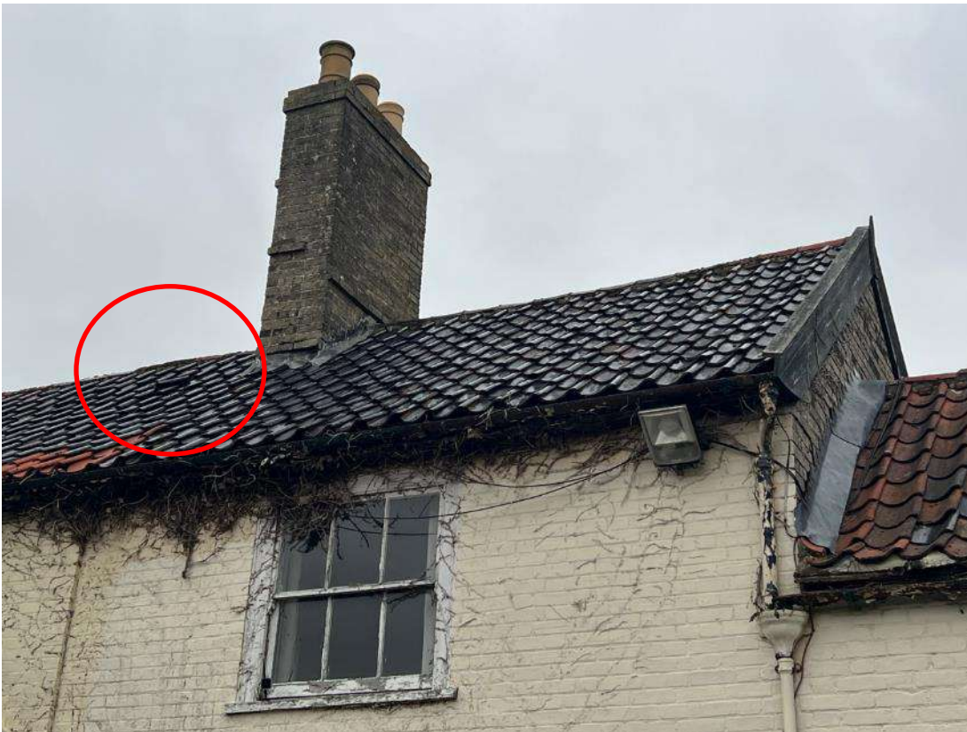
Photo 8. Building 2 (ref B2A). Shows some slipped pan tiles as outlined in red. Evidence that this part of the building was covered with a climbing plant. This has caused damage to the fascia, soffit and under felt.
