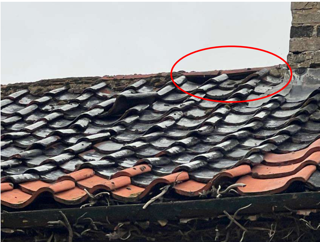
Photo 9. Building 2 (ref B2A). Close up of roof as shown in photo 8. Shows missing mortar under ridge tiles as shown in red.
