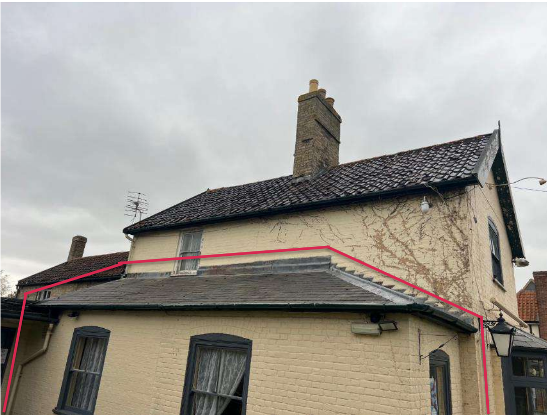
Photo 10. Building 2 (ref B2A and B2B). Shows evidence of climbing plant on side of building B2A. Building B2B is identified by the red outline.
