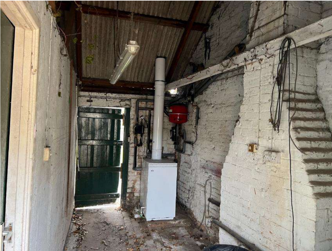
Photo 24. Building 4 (ref B4). Internal view, looking towards western access point. Shows no underlay material.
