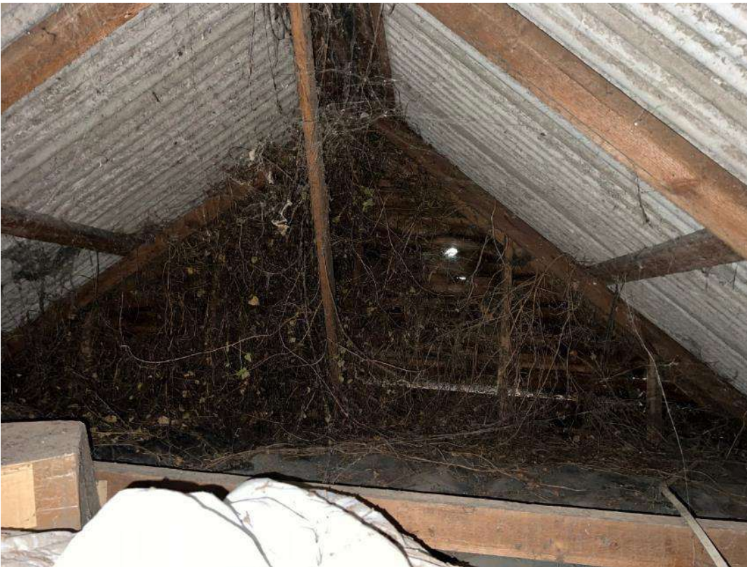
Photo 25. Building 4 (ref B4). Internal view, looking towards southern gable. Shows dense ivy growth within roof space and exposed corrugated sheeted roof.
