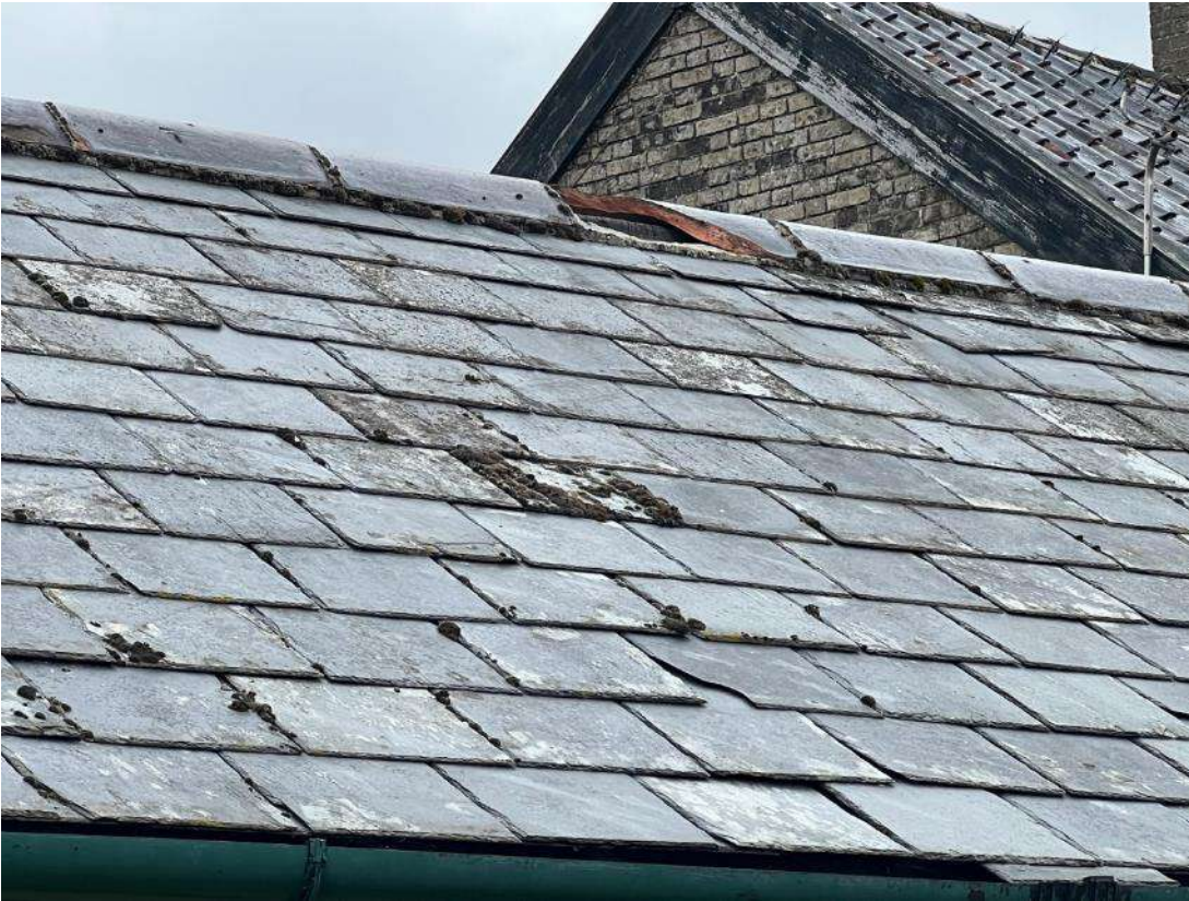
Photo 27. Building 5. Shows close up of damaged ridge tile identified in photo 26.
