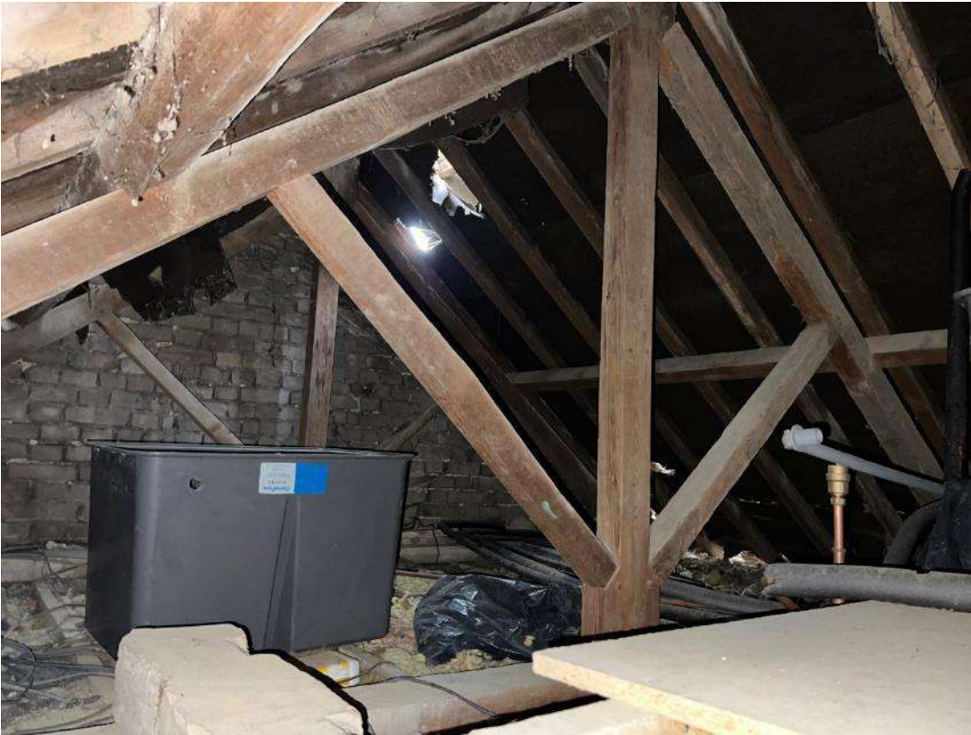
Photo 12. Building 2 (ref B2A). Interval view of roof space. Shows damaged under felt and fire wall between building B2A and B3A. Taken from loft hatch.
