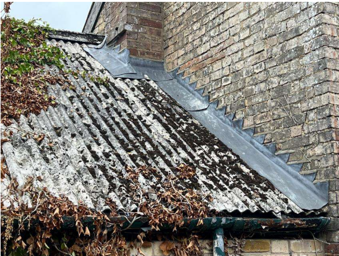
Photo 23. Building 4 (ref B4). Shows gaps between roofing material and brick work. There are also gaps under corrugated ridge.
