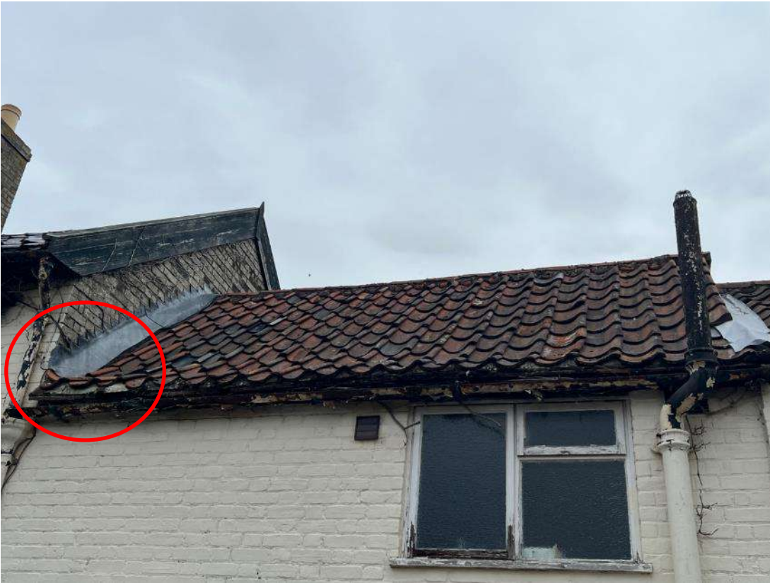
Photo 16. Building 3 (ref B3A). Shows gap under lead flashing where building B3A adjoins building B2A as identified by red circle. Most of the gaps beneath the pan tiles are all mortar filled. West aspect.
