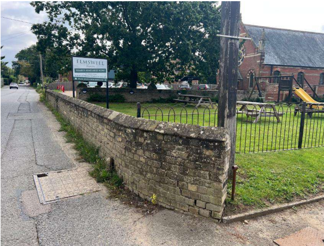
Photo 39. Shows brick wall alongside road and grassland area 1. The oak tree (T3) on the adjacent land is also shown.
