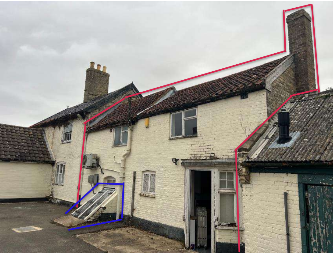
Photo 15. Building 3 (ref B3A). West aspect of building. Extent of building 3 is outline in red. Cellar hatch and loading ramp is identified in blue.
