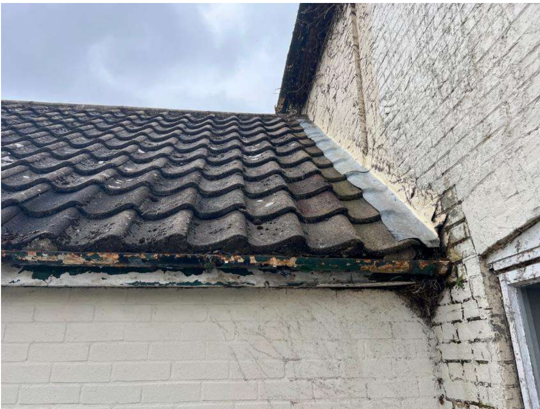
Photo 4. Interface between building 1 and building 2. Gap under lead flashing and damaged barge board. Evidence that this section of the building was recently overed in a climbing plant.
