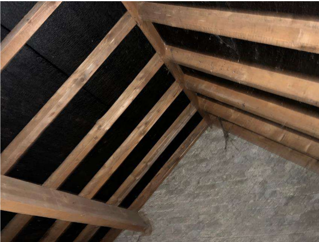
Photo 7. Building 1. South end of roof space. No access points between building 1 and 2.
