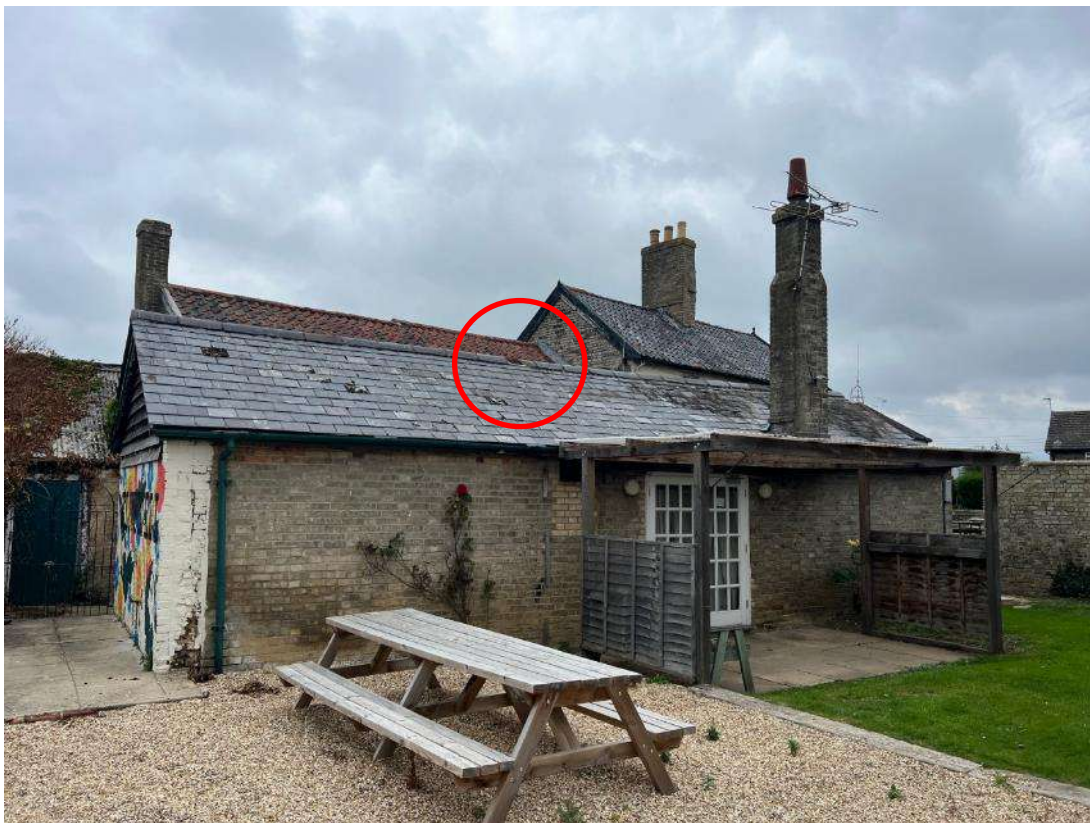
Photo 26. Building 5. Shows eastern aspect of building along with pergola and patio area. Red circle outlines damaged ridge tile.
