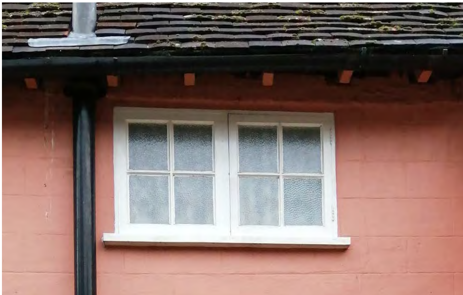
Window WF10 viewed from the exterior (to be replaced).
