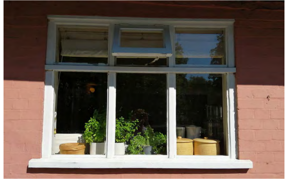
Window WG01 viewed from the exterior (to be replaced).
