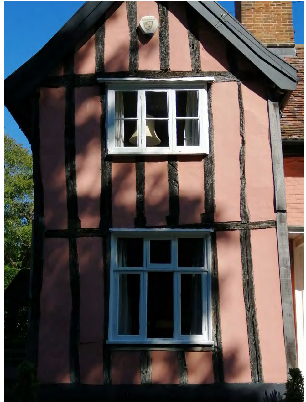
Western crosswing viewed from the south, showing 19th Century window WF04 above (to be retained without alteration) and window WG04 below (to be replaced).
