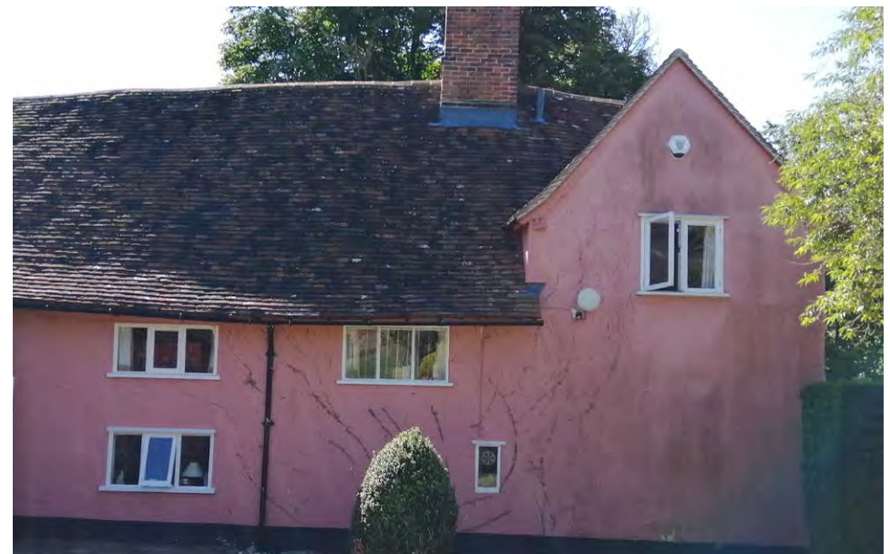
North elevation of Jackdaws Ford showing western crosswing and central hall windows. All of these windows are proposed to be replaced.
