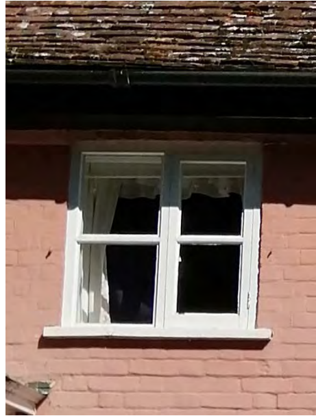
Window WF03 viewed from the exterior (to be replaced with a double casement w/o mullion).
