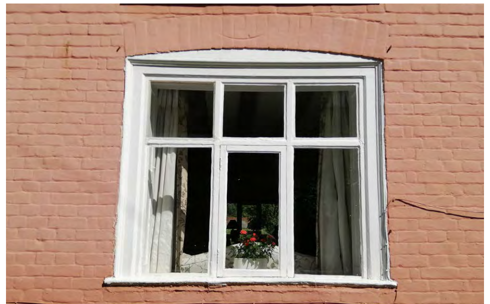
19th Century window WG02 viewed from the exterior (to be retained without alteration).
