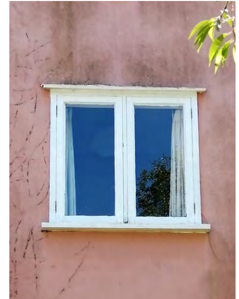
Window WFO6 viewed from the exterior (to be replaced).
