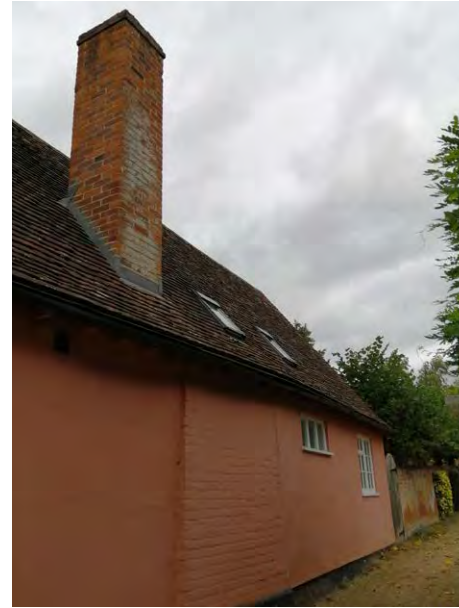
East elevation of Jackdaws Ford showing 'north wing' windows to be replaced
