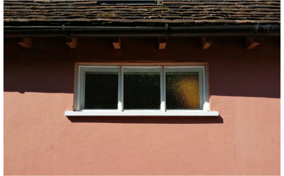
Window WG14 viewed from the exterior (to be replaced).
