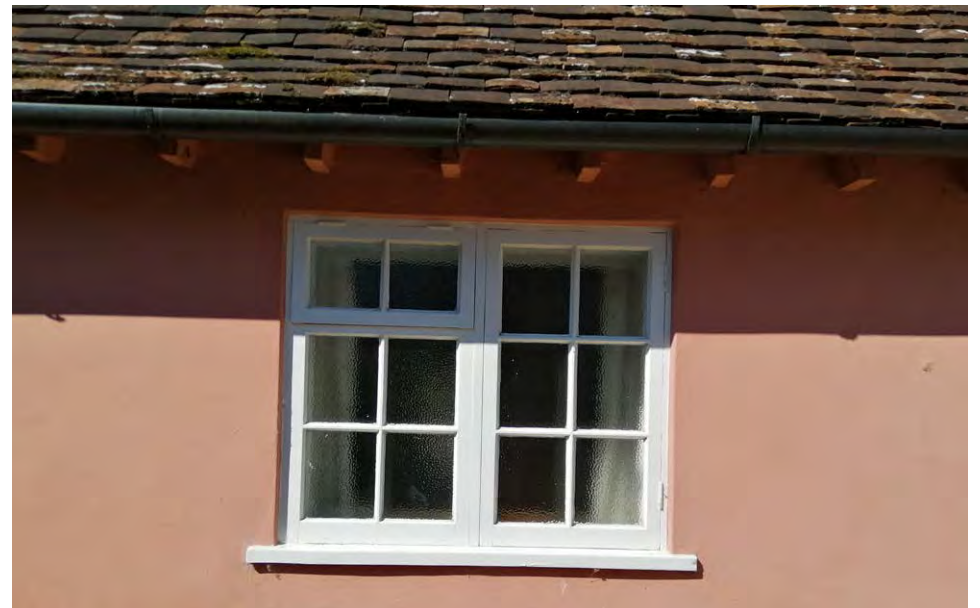
Window WG13 viewed from the exterior (to be replaced).
