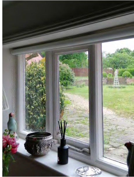
Window WG07 viewed from the interior (to be replaced).
