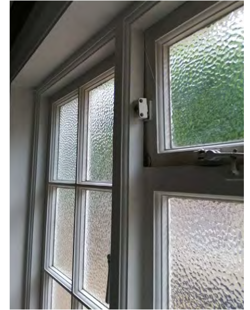
Window WG15 viewed from the interior (to be replaced).
