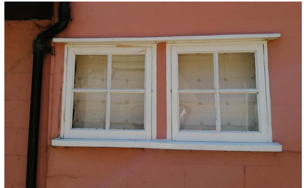
Window WG18 viewed from the exterior. It is proposed to retain the existing structural mullion, frames, cill, and pentice, but to replace the casements with slimline double-glazed casements.
