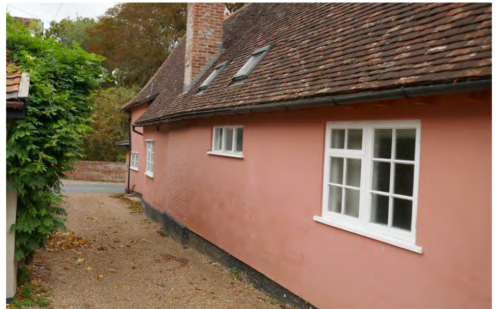
East elevation of Jackdaws Ford viewed from the northeast, showing 'north wing' windows to be replaced. WG13 is in the foreground and WG14 is in the centre of the photo.
