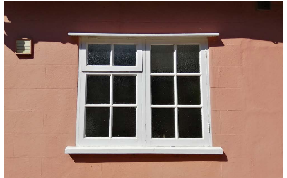
Window WG15 viewed from the exterior (to be replaced).
