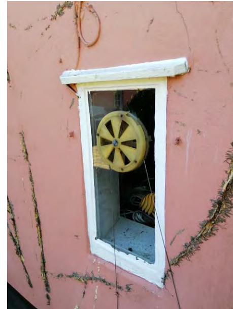
Window WGO6 viewed from the exterior (to be replaced).
