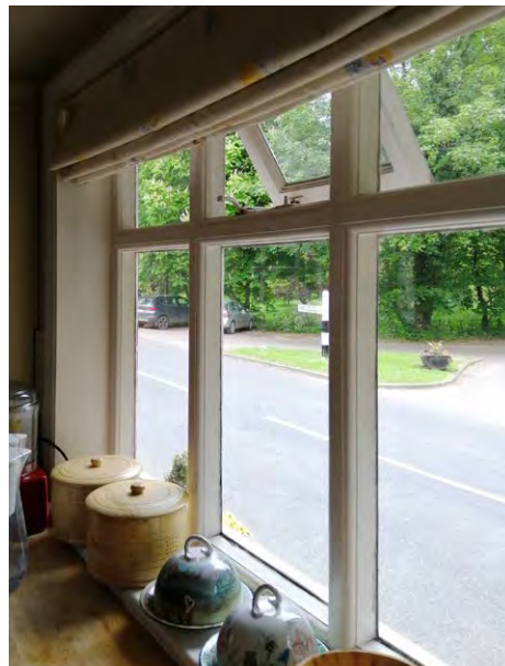
Window WG01 viewed from the interior (to be replaced, fixed/operable layout to be replicated).
