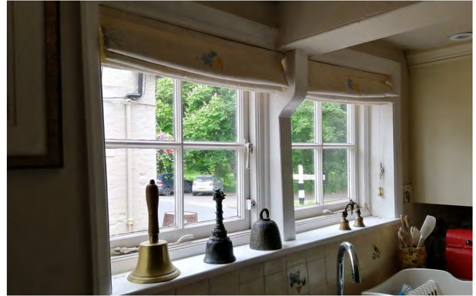
Window WG18 viewed from the interior. It is proposed to retain the existing structural mullion, frame, cills, and windowboards, but to replace the casements with slimline double-glazed casements.
