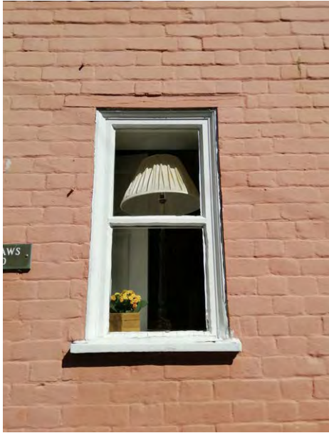
Window WG03 viewed from the exterior (to be replaced, exterior moulding to be replicated).
