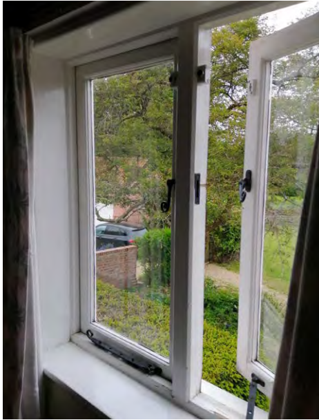
Window WF06 viewed from the interior (to be replaced with double casements w/o central mullion).
