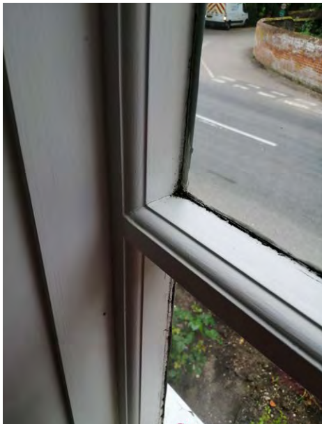
Window WG03 viewed from the interior (to be replaced, central bar profile to be replicated)
