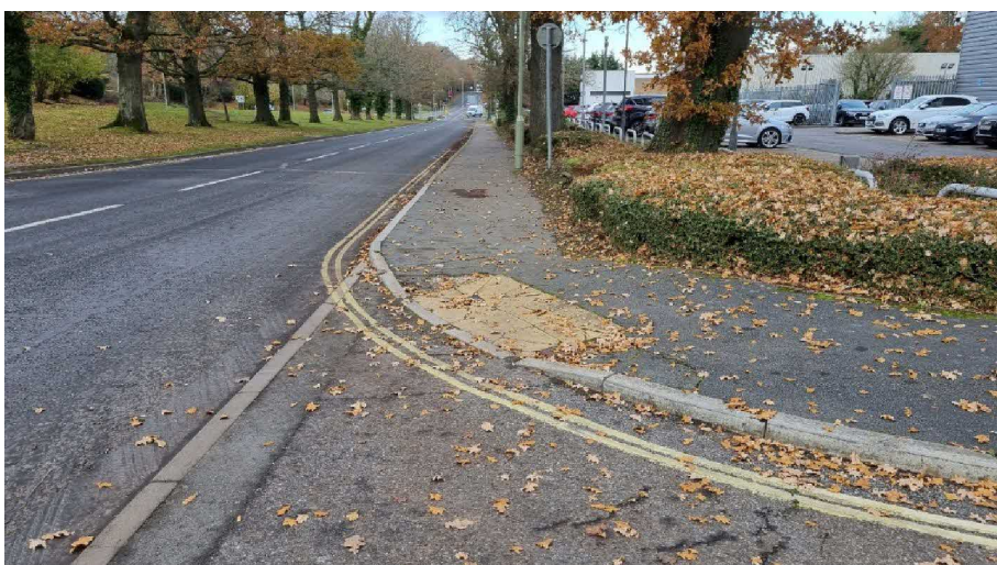
Photo 22: Crockford Lane looking north, mis-aligned tactile paving
