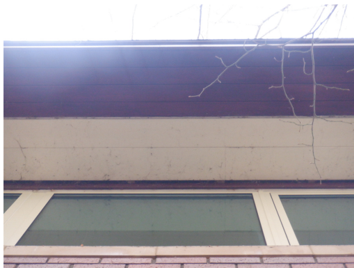
15. Black mesh material between the timber soffit and the wall, viewed on Building 4 from the north.
