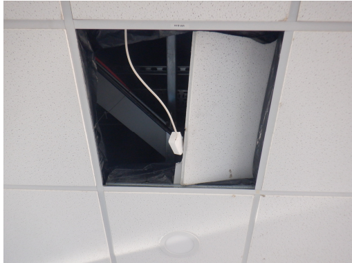
9. Damaged section within the false ceiling of Building 1, allowing partial access to the void above.
