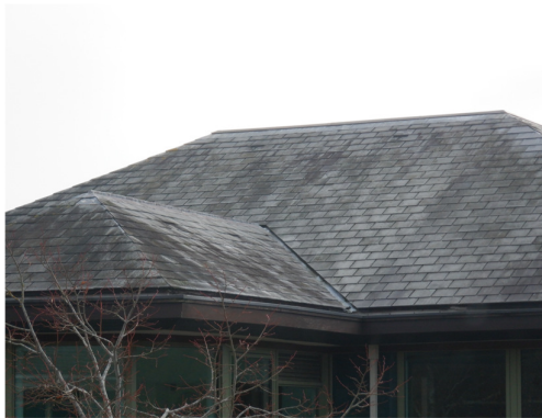
5. Lead flashing between hipped roof and flat roof tight to the slate tiles on Building 1, viewed from the north.
