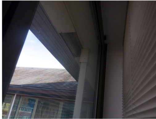
8. Open gap within the timber soffit on Building 1, viewed from the west.
