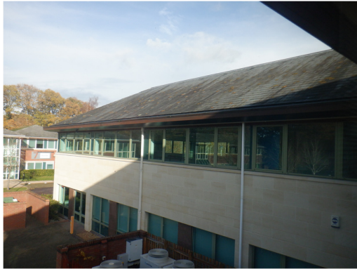
7. Edge of the roof capped off with an underlying metal plate on Building 1, viewed from the southwest.
