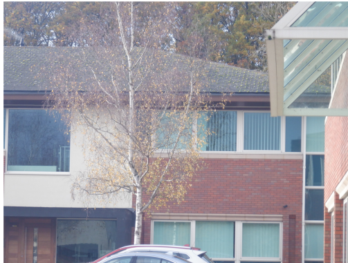
14. Ridge and hip tiles tight to the adjoining slate roof tiles, viewed on Building 3 from the east.
