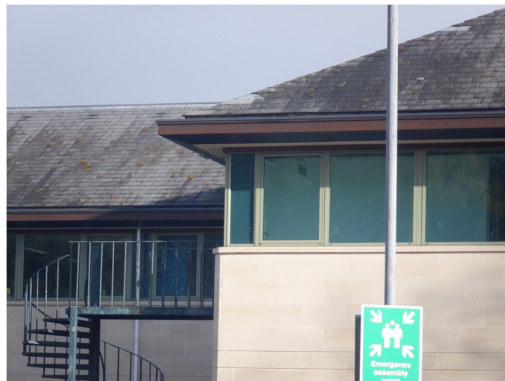
4. Lead flashing under missing hip tiles on Building 1, viewed from the west.
