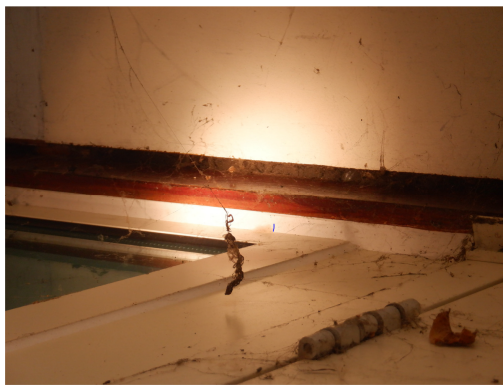
16. Black mesh material between the timber soffit and the wall, viewed on Building 4 from the north.
