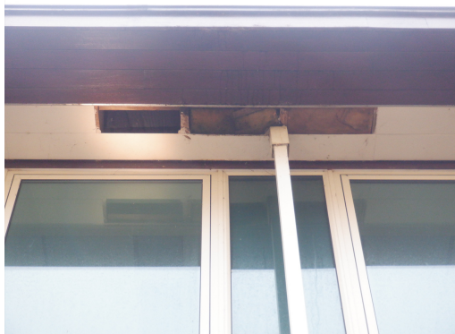
17. Open gap within the timber soffit of Building 4, viewed from the north.
