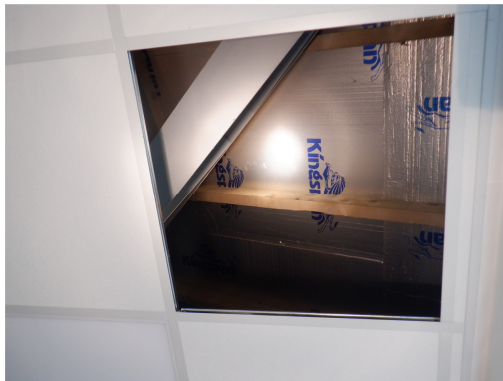
18. Damaged section within the false ceiling of Building 6 allowing partial access to the void above where foil-covered insulation boards are tight to the timbers.
