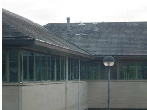
6. Tight lead flashing under flue pipes on Building 1, viewed from the north.
