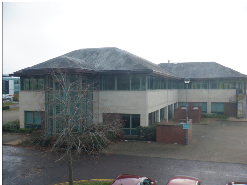
3. Occasionally missing slate roof tiles on Building 1 with superficial crevices, viewed from the north.
