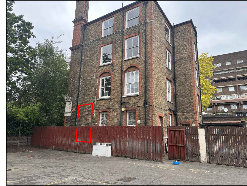
Wall Mounted ASHP Location
