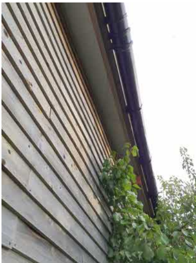
Plate 3: Indicative image of cladding showing lack of gaps and good condition of soffit boxes
