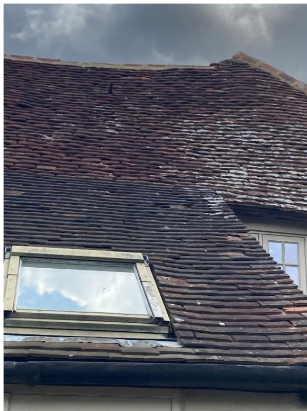
Photograph 4: Area of the inaccessible partitioned loft with lifted tiles present
