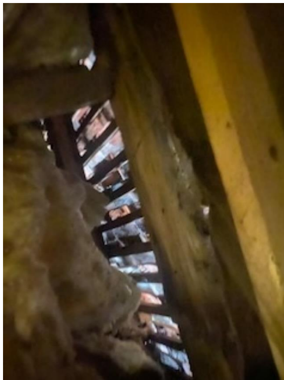
Photograph 2: Day light visible due to no roofing felt present in partitioned part of the loft
