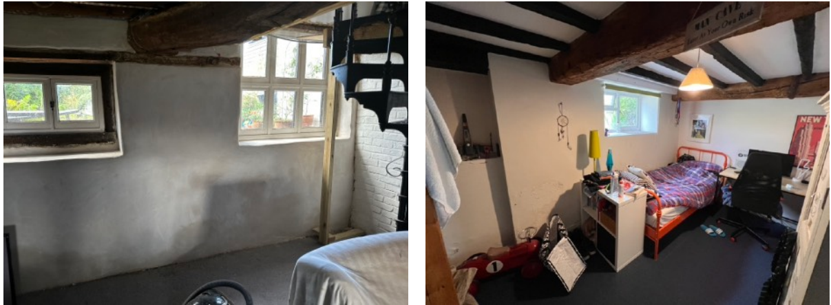
Fig 2. Existing Living Room showing internal lime rendered semi-basement wall along back of house and Fig. 3 failing concrete tanking system, to be removed and lime rendered.
