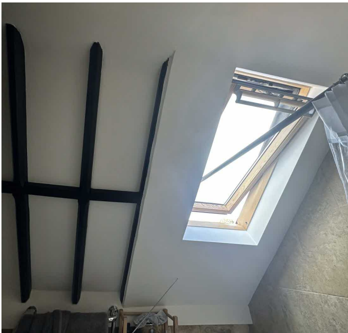
Figure 3: Inside—main bathroom existing rooflight. Proposals to achieve similar outcome in adjacent en-suite
