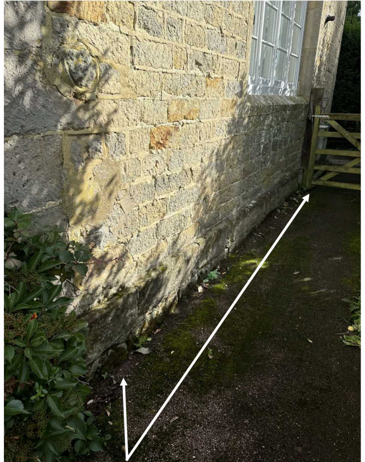
Figure 5: West elevation of house where gravel trap to be installed along side of building and tarmac cut back away from building
