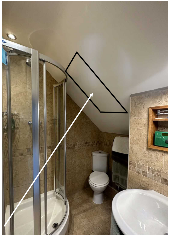
Figure 4: Inside—existing en-suite. Proposed to install new rooflight between 2 existing rafters, only requiring cutting of 1 rafter
