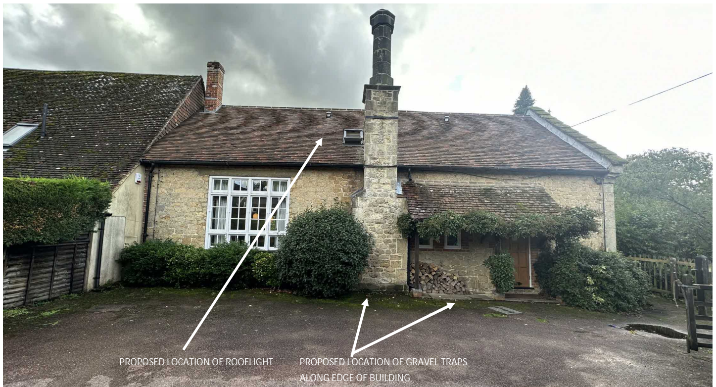
Figure 2: North elevation of house—issues with surface water can be seen by the green moss along the edge of the house & flower beds.
